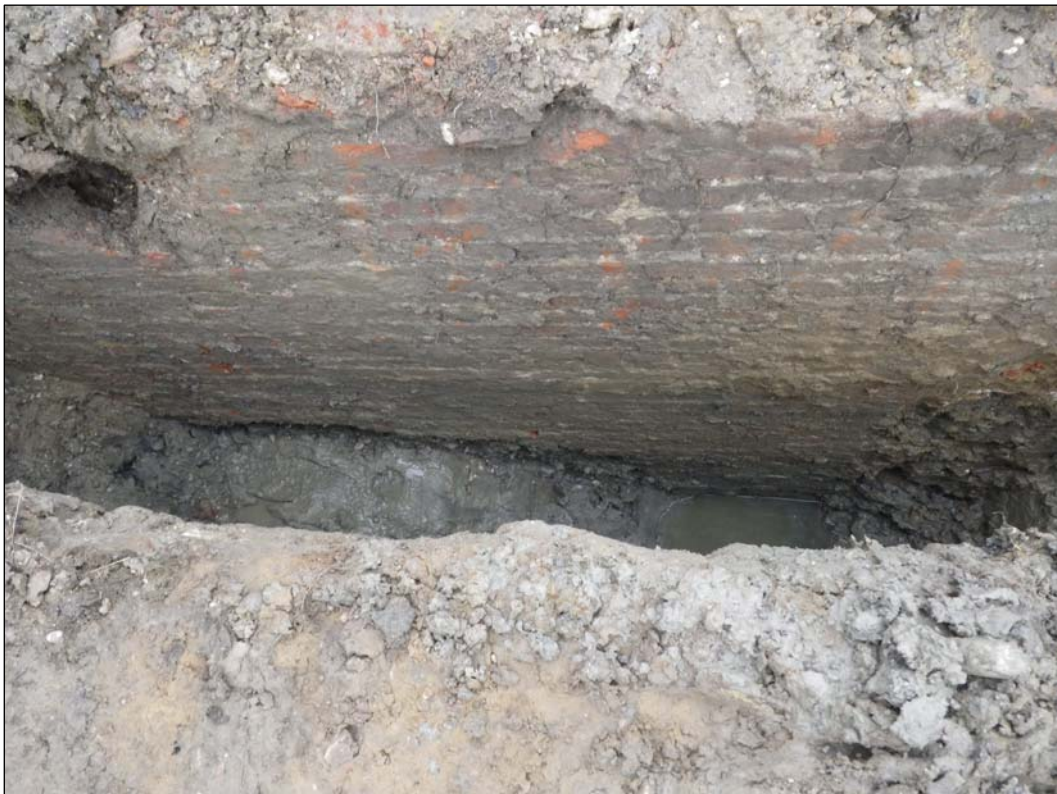
Plate 4. Full depth of the brick wall, immediately south of the arch, showing waterlogged clay through the base.
