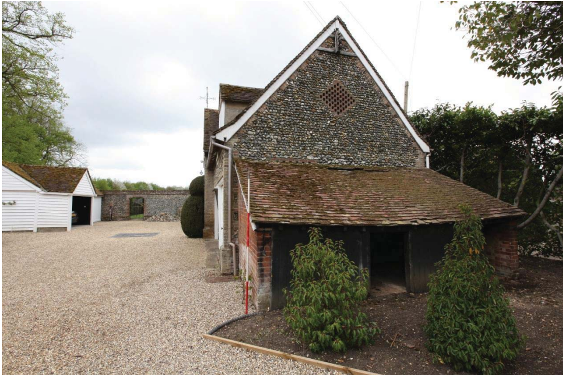
Illus. 7. The eastern external gable with a diamond-shaped pattern of ventilation bricks to the loft and a rectangular pattern to the former eastern stable (the latter just visible above the roof of the later lean-to log store which bears the incised date 1901).
