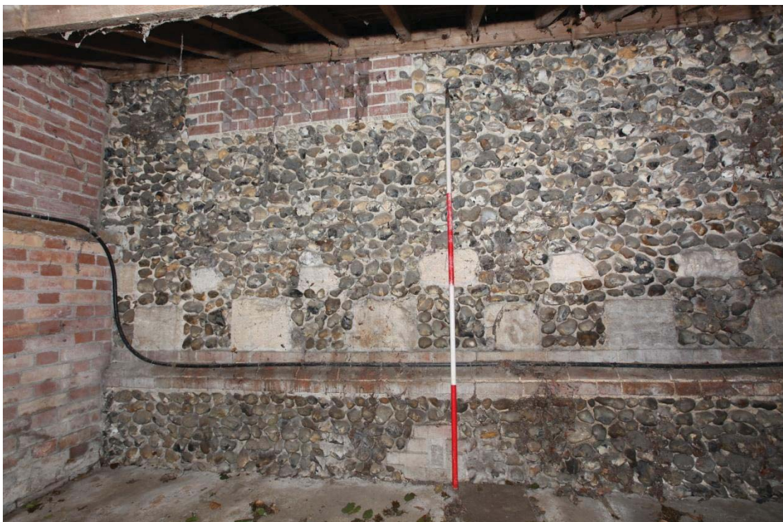
Illus. 8. The lower part of the eastern external gable seen from the later log store. The rectangular-shaped pattern of ventilation bricks is visible top right, with a blocked drain serving the former eastern stable below. The irregular chequer-board pattern above the plinth consists of large re-used blocks of masonry that may have been salvaged from the parish church in 1854 and suggest a possible date for the building.
