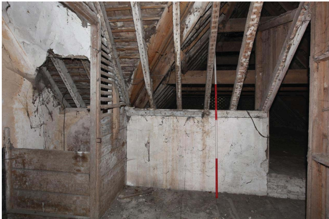
Illus. 14. The interior of the attic above the coach house seen from the west, with the boarded chaff box at the head of the stair to the left and the secondary doorway to the loft over the eastern stable (now the garage) on the right. The attic was originally fully plaster with a ceiling at collar height and extended from the stair to the front (southern) gable.
