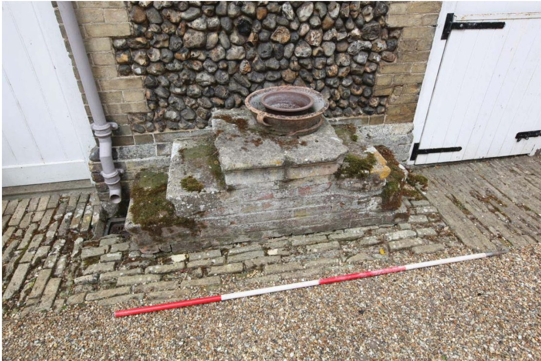
Illus. 5. The brick mounting block with moulded stone steps to the left of the entrance to the western stable. The gault-brick dressing behind the drain pipe marks the south-western corner of the original building.
