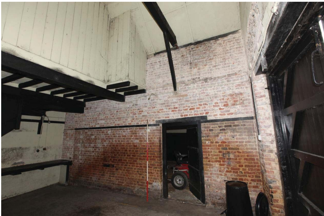
Illus. 10. The interior of the central coach house from the west showing the door to the garage and the remains of the ceiling. This ceiling originally continued to the southern gable on the right but was later removed to increase headroom. The scar and wooden support of the missing principal joist is visible above the door and beneath the later brace to the tie-beam.
