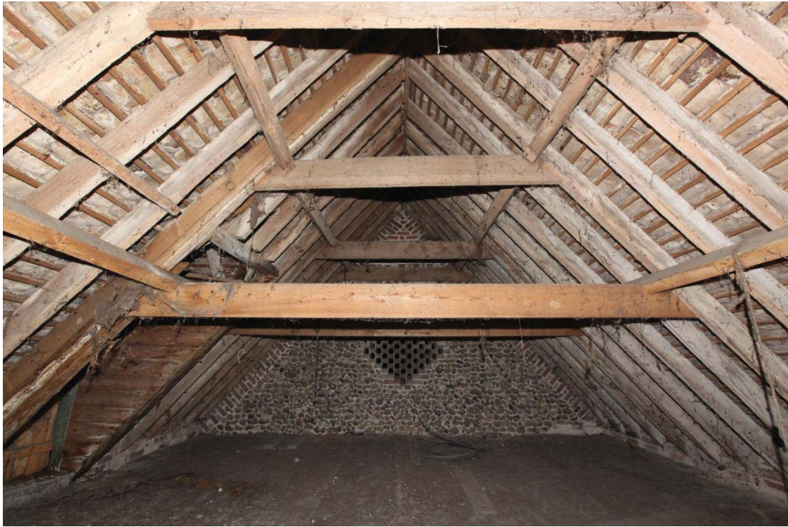
Illus. 15. The interior from the east of the loft above the western stable showing the ventilation diamond in the original western gable (now blocked by the tack room extension). The higher collars and purlins are original to the roof structure but the lower tier of light-coloured pine is a secondary insertion; the original collars are tenoned and pegged to the rafters while the secondary collars are nailed.
