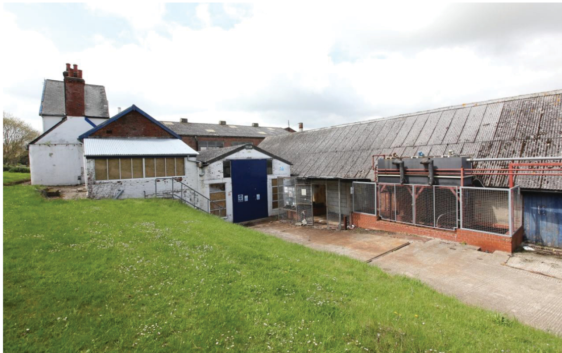
Illus. 4. The exterior of the complex from the east showing the corrugated asbestos roof of the yarn store to the right (a 19 th century single-storied brick shed, the southern elevation of which was rebuilt in cement blocks during the 20 th century). The roof of the dye house is visible in the rear with the narrow dwelling house on the left and the gables of the drying room (with blue doors) and the lab (with glazed lean-to) in the foreground.
