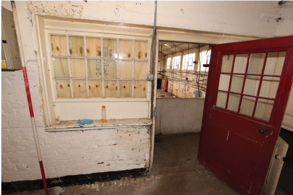
Illus. 11. The 19 th century door and window opening from the office floor into the southern gable of the dye house at the eastern end of the passage behind the WCs. Both features appear to interrupt the brickwork and may be secondary.
