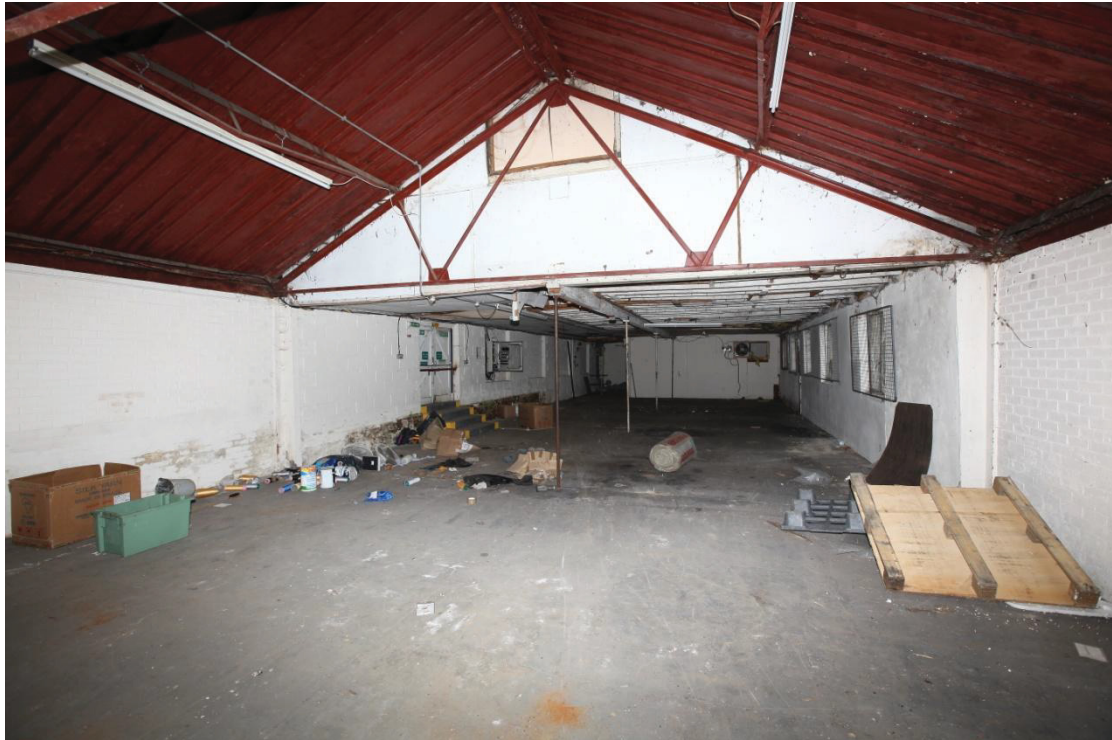
Illus. 9. The yard store from the eastern gable of its 20th century extension (to the left in illus. 5) showing the remains of the original 19 th century gable supported by an iron post in the centre. There is evidence of a series of 19 th century windows in the northern elevation on the right but the southern wall has been rebuilt above its red-brick plinth.
