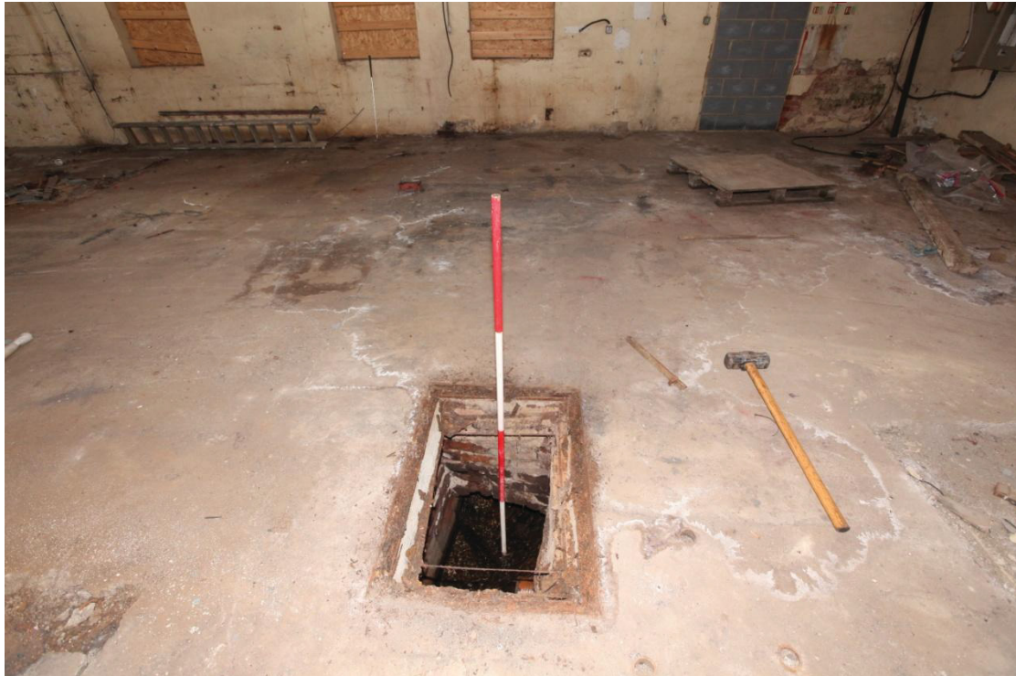
Illus. 7. The concrete floor of the dye house viewed from the east showing the man-hole opening onto the fast-flowing water of the 19th century mill stream which still flows beneath the building. There is no obvious evidence a wheel pit or any other original mechanism, and this probably represents the by-pass channel.
