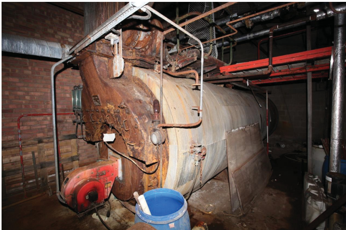
Illus. 10. The substantial mid-20 th century boiler in the 'old boiler room' of Fletton brick seen from the north-west.
