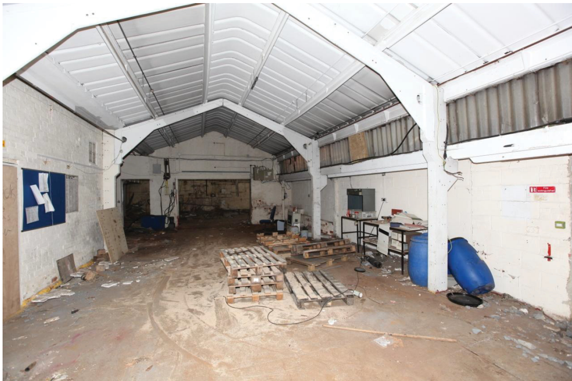
Illus. 8. The steel and concrete-framed 20th century shed which operated as a drying room, with the entrance to the dye house in the rear. The door on the left opens onto the cellars beneath the lab and the wall on the right (largely rebuilt in cement blocks) is part of the 19 th century single-storied dye and yarn store.
