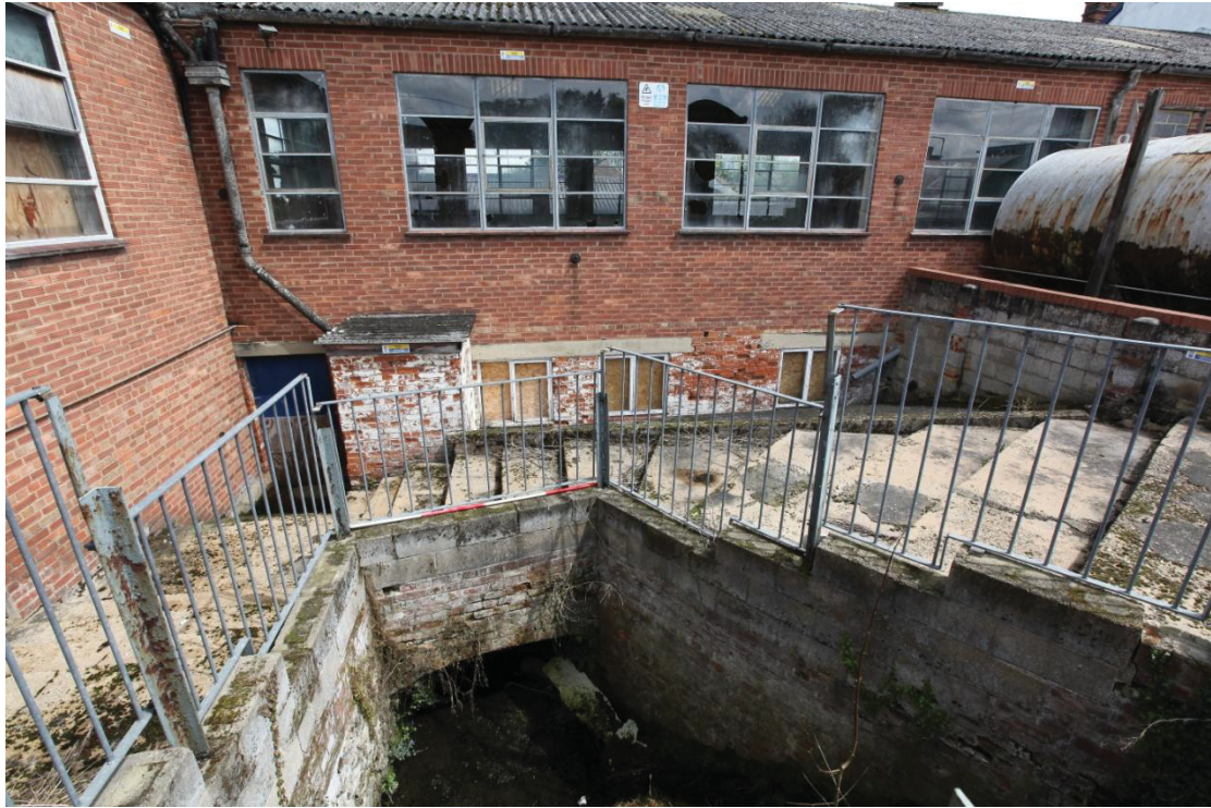
Illus. 3. The 19 th century mill race flowing beneath the dye house, viewed from the site of the headwater pond to the west. The whitewashed red brick beneath the concrete widow lintels survives from the original mill but the rest is a reconstruction of the 1960s when the sheds on the left were added.
