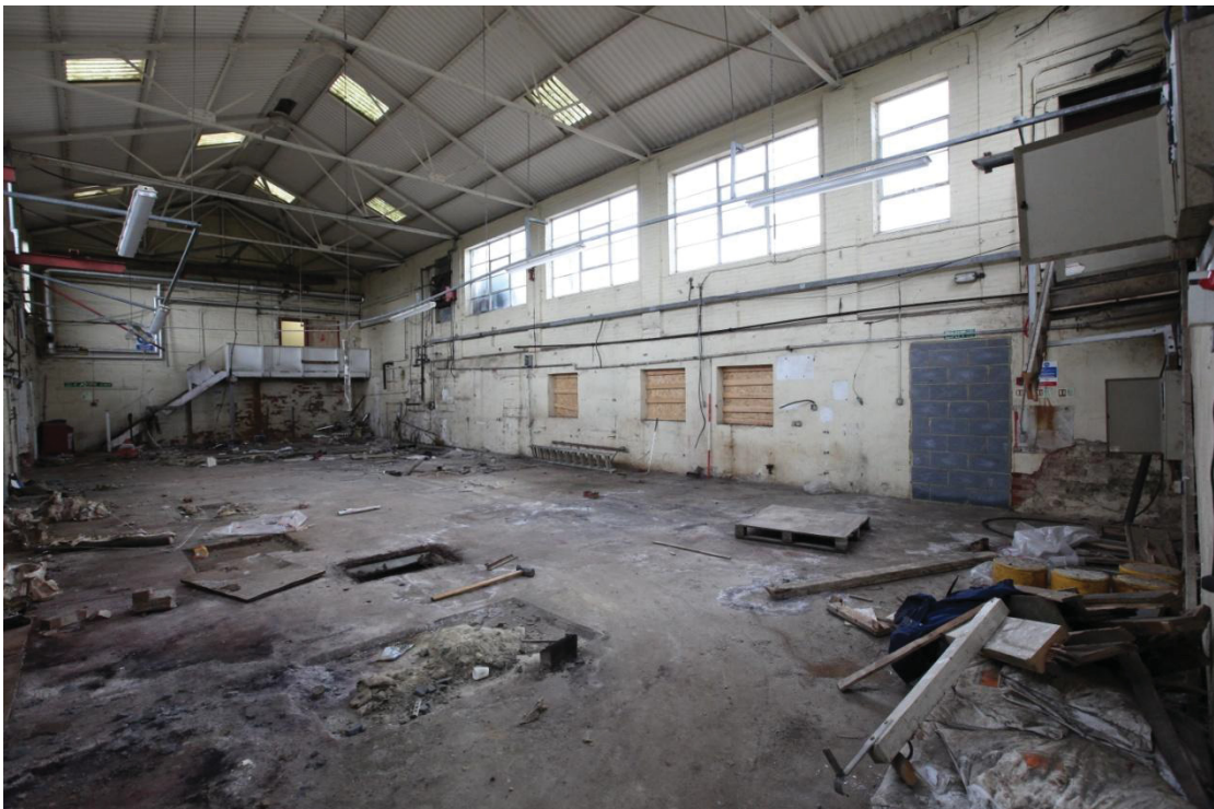
Illus. 6. The interior of the dye house from the north, showing the positions of the removed dye vats in the concrete floor. The stair and gallery projecting from the southern gable in the rear opens onto the office floor, with the scar of an earlier stair belonging to the demolished upper storeys of the mill to its left. The lower walls of this structure survive from the 19 th century but the rest dates only from the 1961.
