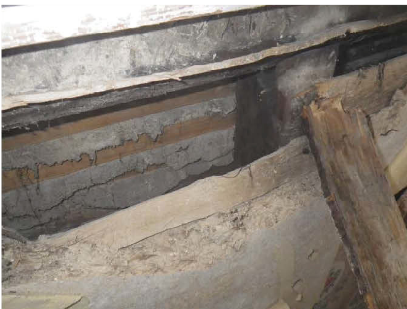
Inside of the front wall in Room F1 showing the timber framing. The vertical stud had been altered possibly to create a larger window opening and there was no indication of medieval carpentry joints. The photo shows the back of the external render which has been replaced in the recent past.
