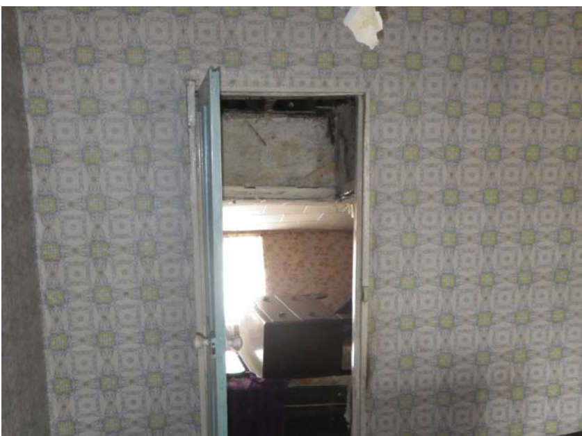
The door between Rooms F1 and F2 at the rear of the house. The floor and ceiling heights are much lower at the rear and a raised box-like section has been built into the rear ceiling to allow passage through the door.
