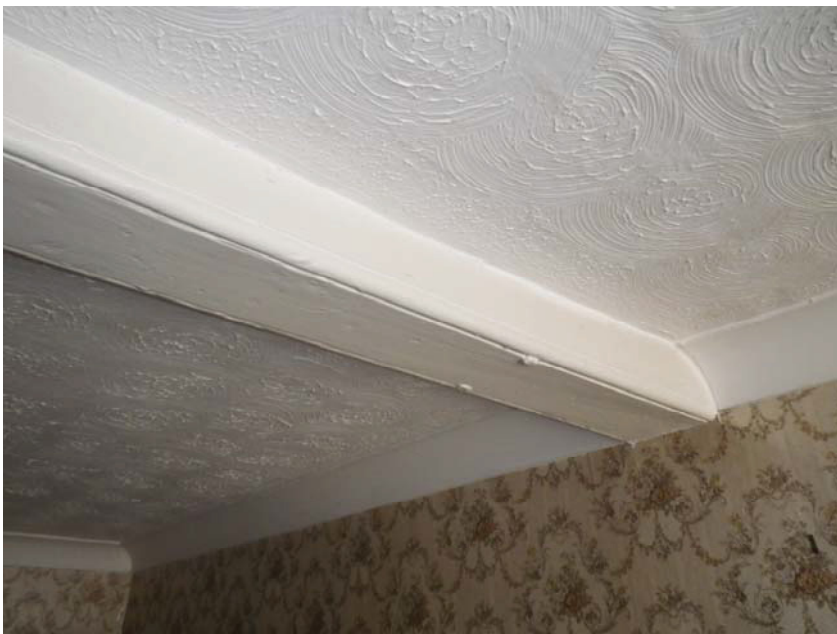
Bridging beam running across the centre of rooms G4 and 5. The moulded corners passed through the partition wall uninterrupted; this is not an indication that the partition is an insertion as there are no moulded stops on the beam ends.
