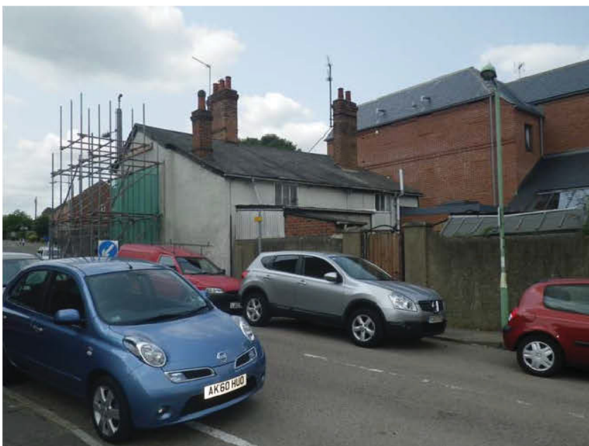
Rear of the building viewed from Duddery Road. The asymmetrical roof and the slight step in the gable wall suggest that the building is built in two bays, the rear being in effect a lean-to. The bays are contemporary.
