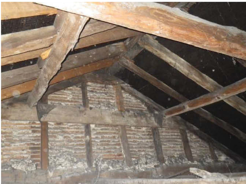
Roof structure over no 87 looking S. with clasped purlins. The purlins and the collar in the immediate foreground are made from timber left in the round; the plank-like collar at the far end is a replacement. Note the large tie beam which seems to have been made from two pieces of wood joined with a half-faced scarf joint. The well spaced studs suggest a late date.
