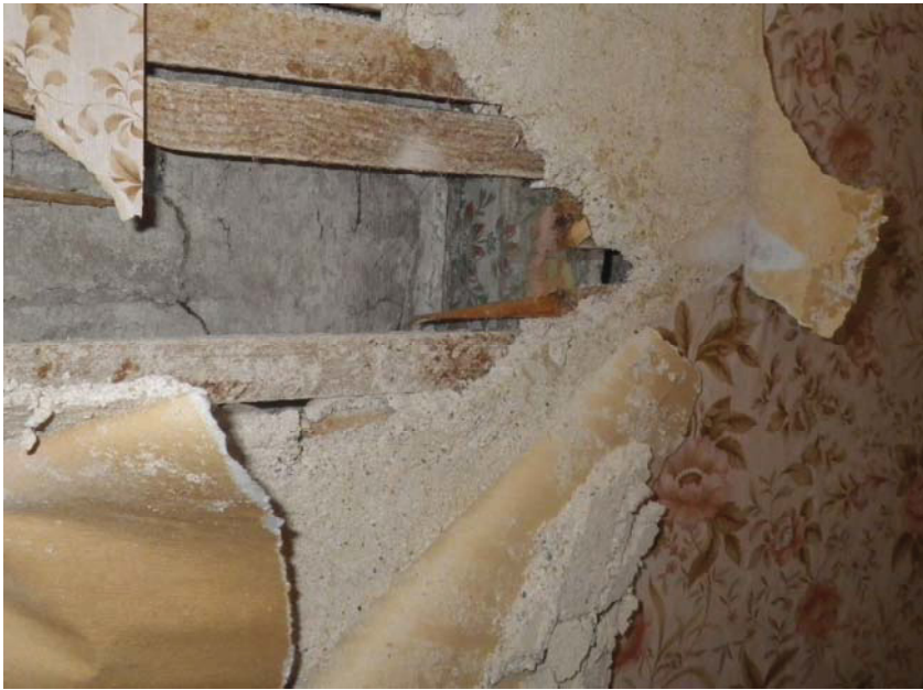
South gable wall in room in F1 showing the original plaster recessed back from the face of the studs behind later plaster work. The now hidden studs appear to have been individually wall-papered in a virtuos display of decorating.
