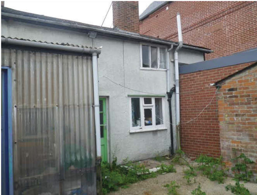
The rear of No 87 viewed from the north. The modern brickwork alongside the soil pipe follows the property boundary as shown on the tithe map of 1840 so that the north end of the building projects into the neighbouring plot in the manner of a flying freehold.
