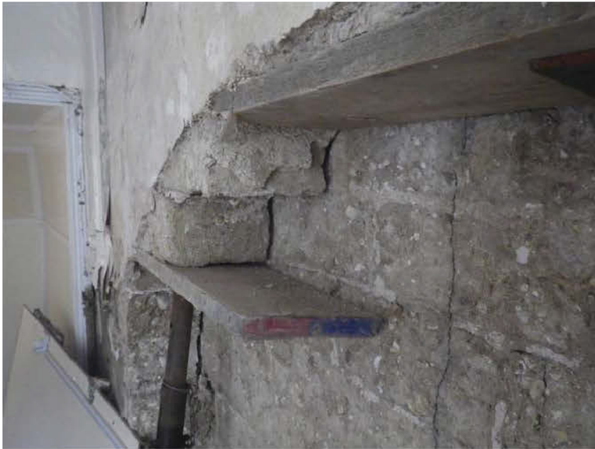
Double skin of clay lump block forming the south gable wall in room G1. The wall changes to timber-frame construction at first floor level. Note that the two faces that make up the wall do not appear to be bonded or keyed together.
