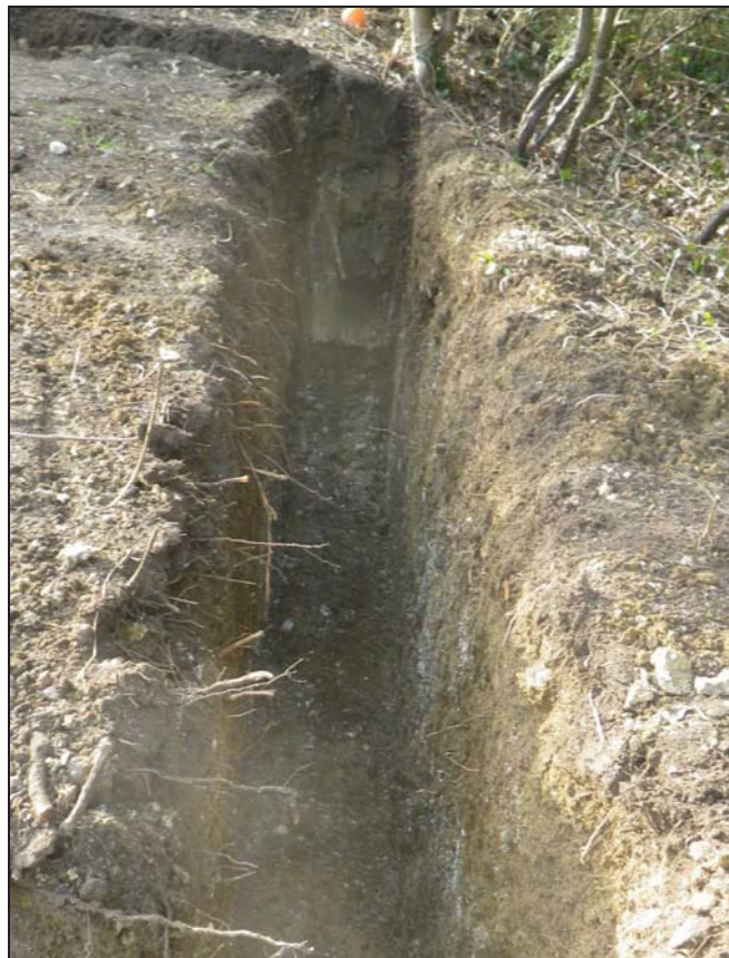
Plate 4. Garage footing with hedge and ditch beyond to the right of the picture (north)
