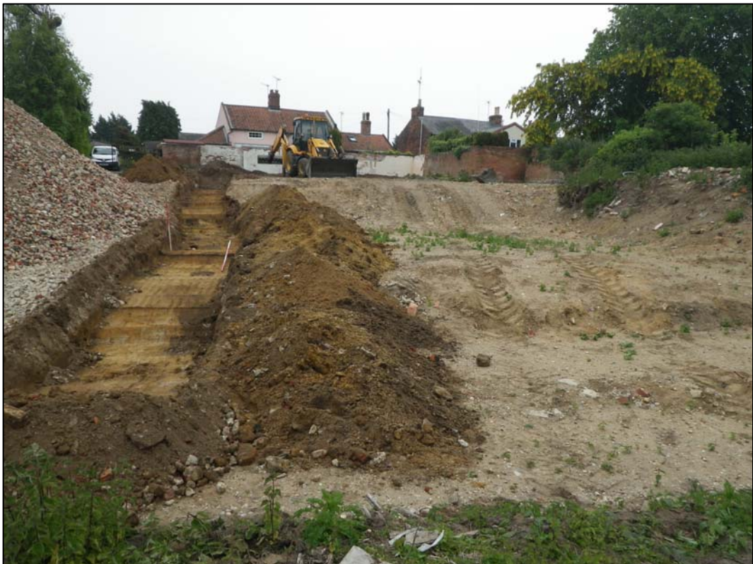
Plate 2. Trench 2 showing the area of the former warehouse, note the variation in levels
