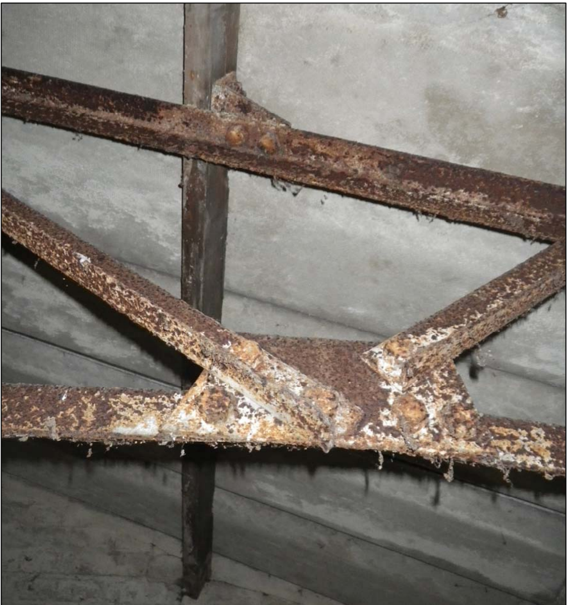
Plate 10. roof truss detail showing bolted plate joints and angled bracket holding a purlin (ref. HTQ 73)
