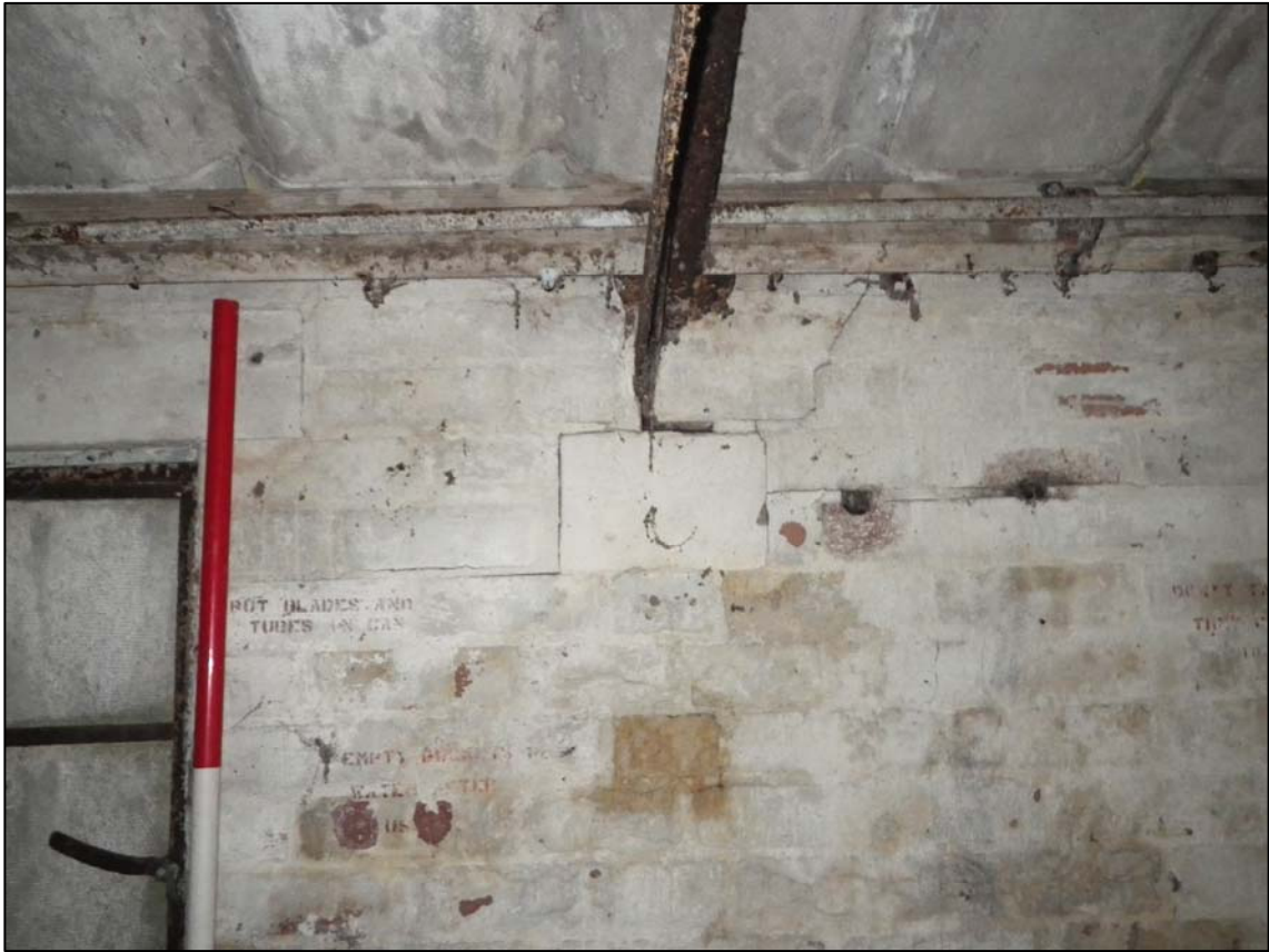
Plate 11. roof truss detail - foot of truss resting on block within wall (ref. HTQ 94)
