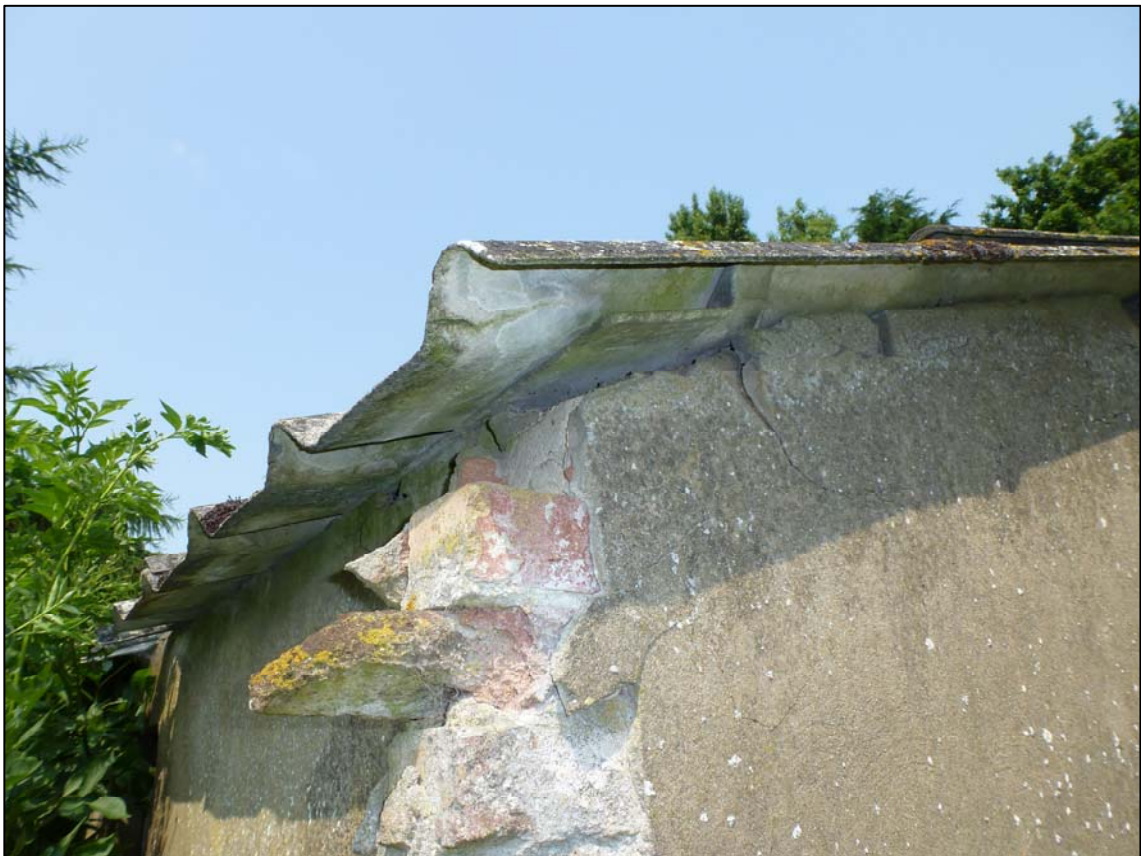
Plate 12. roof detail - shaped fibre board upon which the roof rests (ref. HTQ 44)
