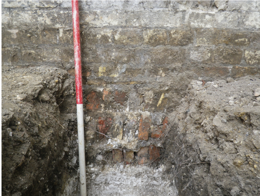
Plate 3. Foundation of Shrublands House made of re-used bricks which date from C15-16th and are in contrast to the gault bricks of the wall above ground. Three courses of bricks (roughly laid with the bricks on edge) make up the foundation which is built directly off the surface of the underlying chalk geology. The footing trench for Shrubland cut occupation/demolition deposits associated with previous occupation of the site (shown below)
