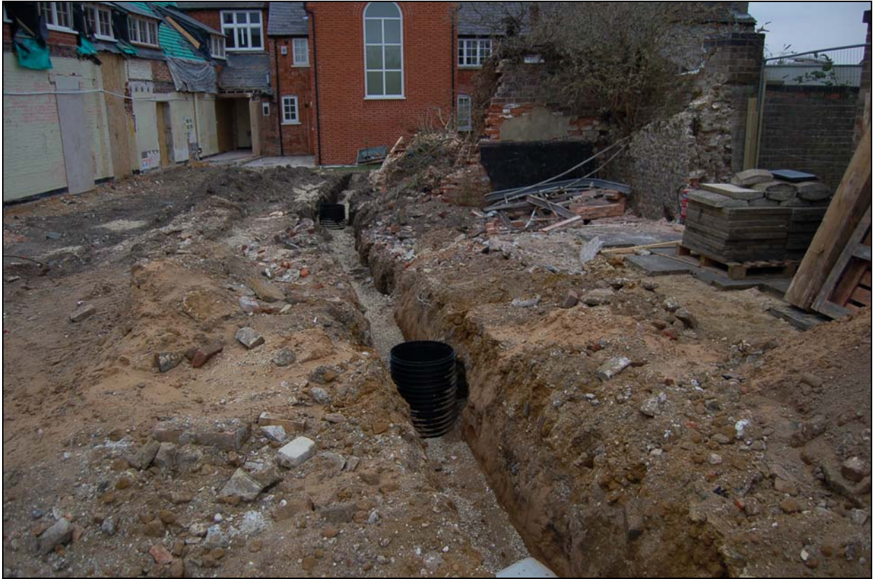
Plate 4. Service run adjacent to new build area (left of shot), facing north
