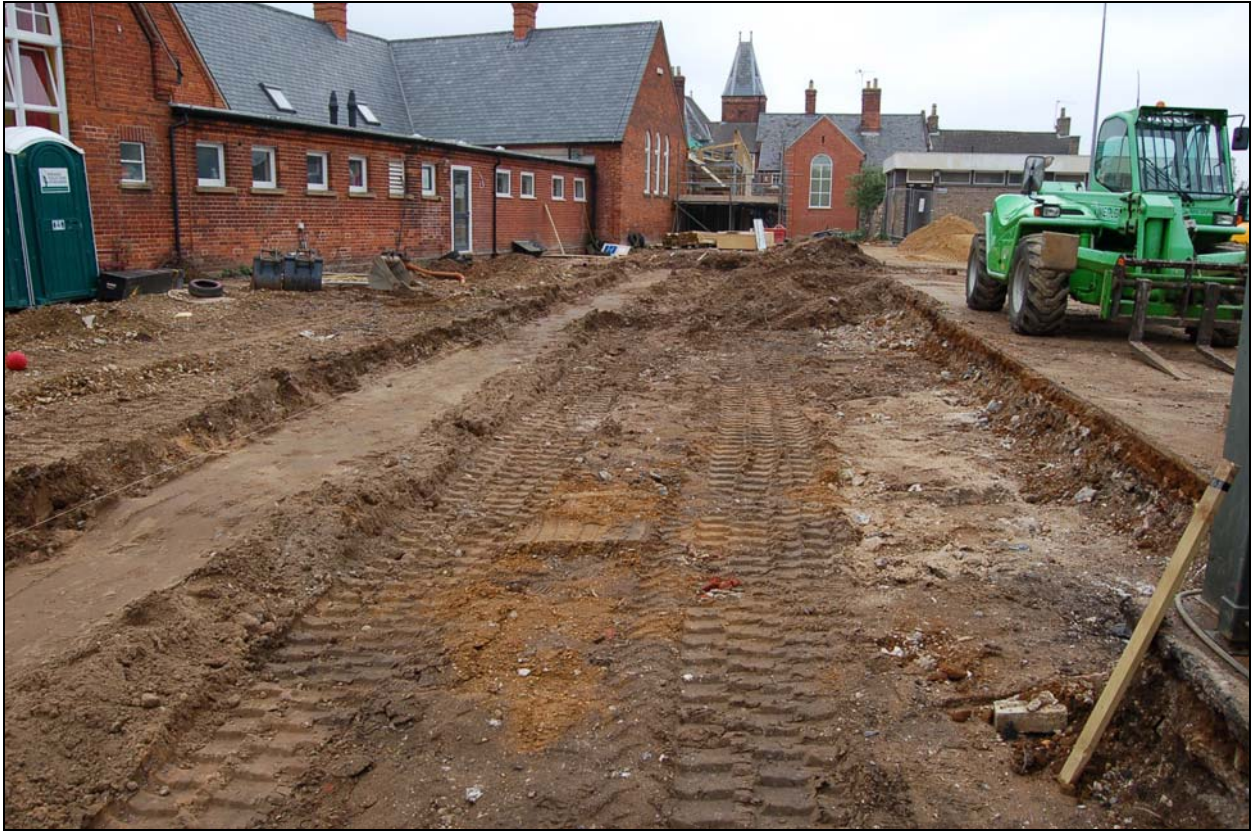
Plate 6. Soak away in car park showing outbuilding foundations (eastern side of soak away), facing north
