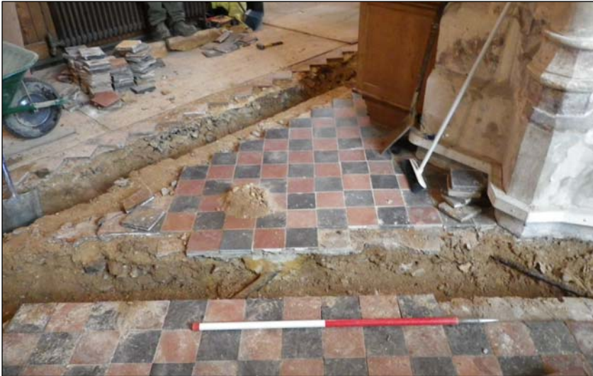
Plate 6. General view of internal service trenches
