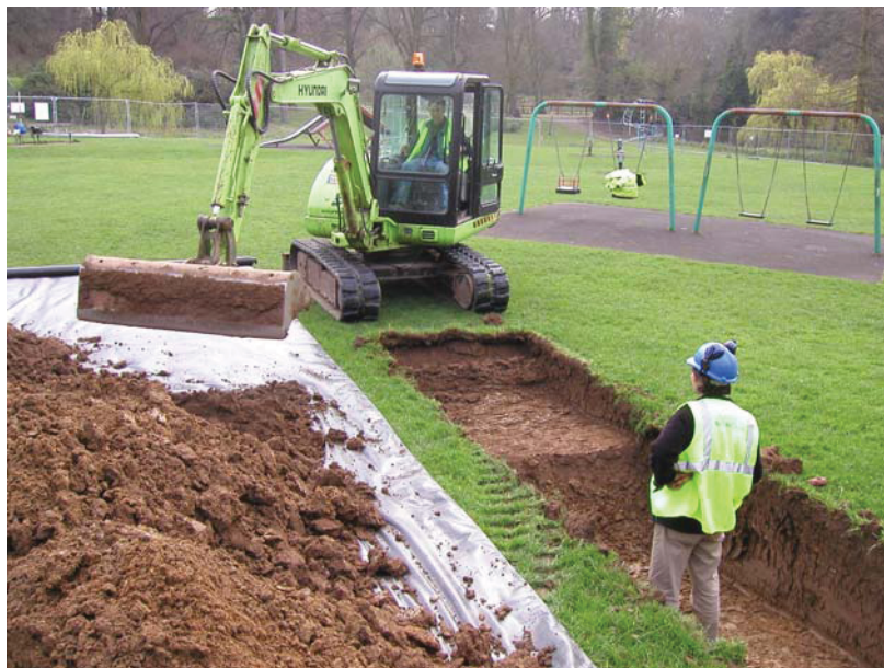
Plate 3: Machine digging trenches, trenches had to be positioned to avoid play equipment.
