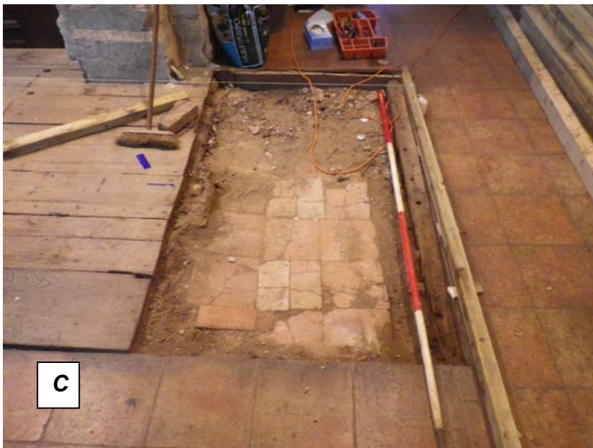
C) Worn floor tiles in the north aisle exposed during repairs to the timber floors. The large tile were unglazed earthenware dating to 16th-18th century. The tiled surface is below the level of Norman stone work at the base of the piers indicating that the floor had already been lowered by the time the tiles were laid.
