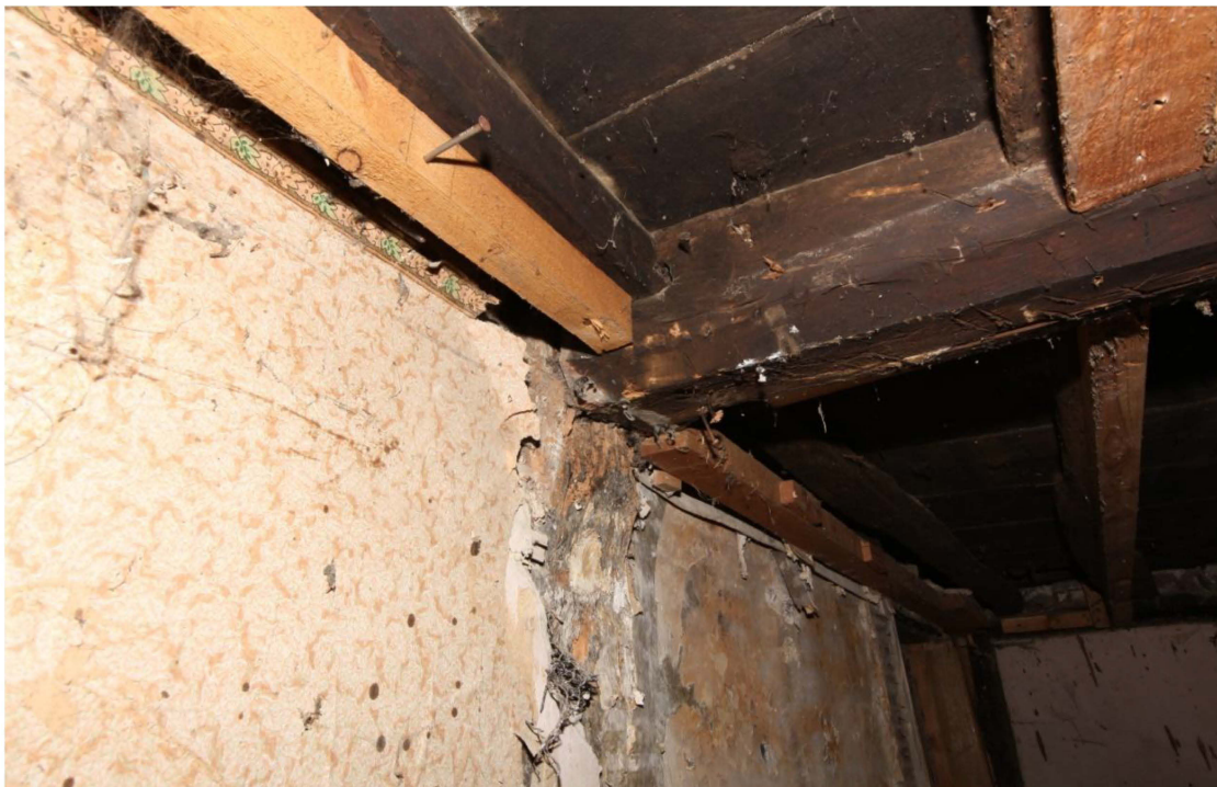
Illus. 20. A detail of the northern gable of the hall from the rear (west) showing the integral corbel block which projects from the central post to support the neatly chamfered axial joist of the ceiling. The common joists are secured by soffit-tenon joints in the typical manner of the 16 th century. The original chamfered clamp of the front wall is visible in the rear.
