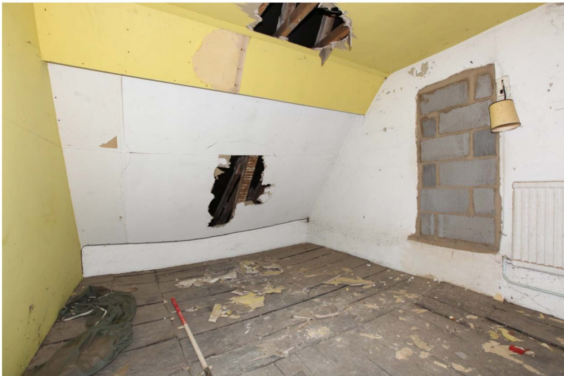
Illus. 12. The northern bedroom from the east showing a blocked door to Pottery House on the right and the unusually complete floor of rebated oak boards. The framing is hidden by late-20 th century dry-lining.
