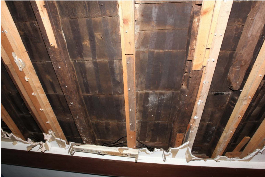
Illus. 11. The hall ceiling from the rear (west) showing a number of recent softwood joists inserted to strengthen the original oak joists which survive largely intact and in good condition along with the original rebated oak floorboards. Both joists and floorboards were heavily and abnormally smoke stained before the application of render to the undersides of the floorboards as indicated by the distinctive pattern of stripes.
