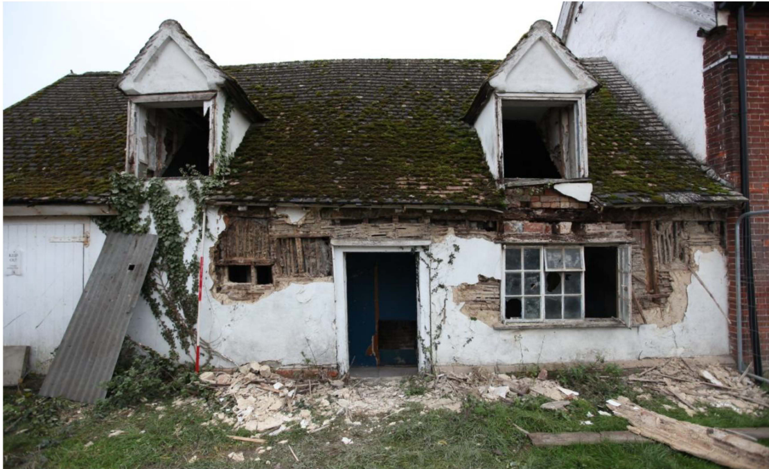
Illus. 15. The eastern facade photographed on 3 rd December 2013 after the partial removal of the render shown in illus. 3 above. The original roof-plate, studs and internal braces proved to be largely intact with substantial areas of wattle-and-daub. Note the window lintel to the left of the entrance.
