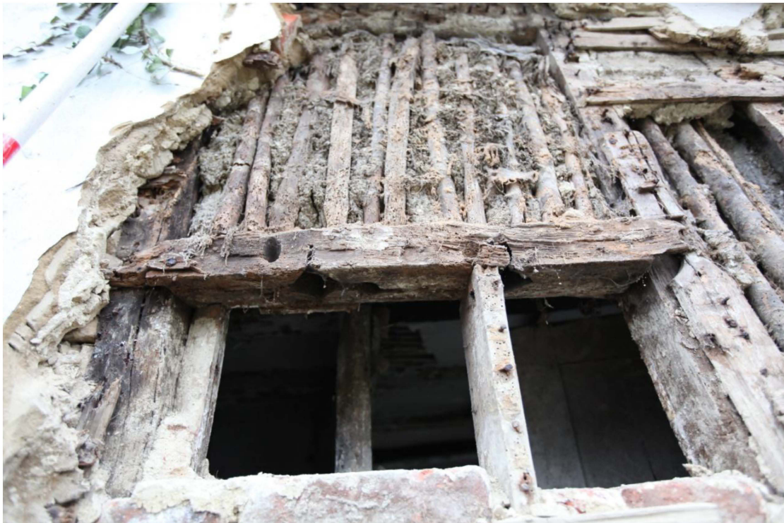
Illus. 16. A detail of the original window lintel to the left (south) of the entrance door in the eastern facade with two diamond mullion mortises in its soffit. The sill has been removed but its pegged mortises remain in both jambs. The lintel has been damaged slightly but still overlaps these jambs and would have projected through the original external daub. It contains two dowel holes angled upwards at approximately 45 degrees that may have supported an external drip board or hood to exclude rain in the absence of glass.
