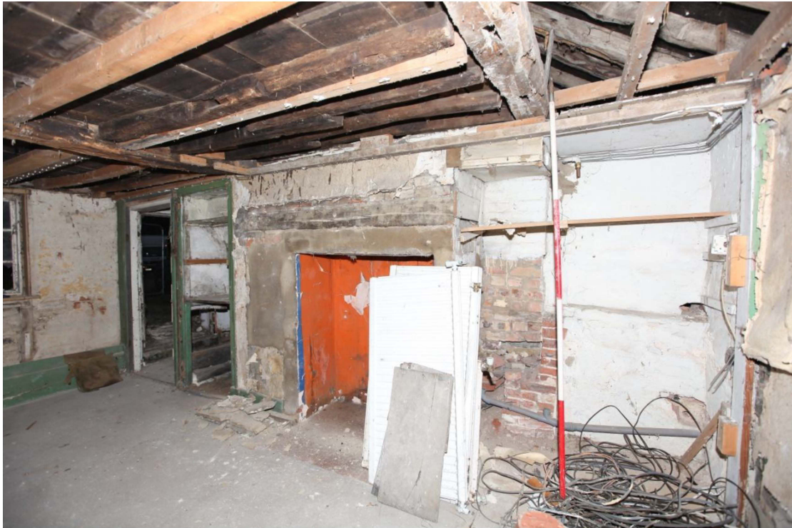
Illus. 17. The newly exposed fireplace in the hall with a large timber lintel that formerly extended to the rear wall – the position of which is indicated by the scale rod. The timber supporting the original ceiling joists was inserted when the lean-to extension was added and the wall removed; it contains stud mortises but has been re-used from elsewhere. The original roof-plate survives immediately above.
