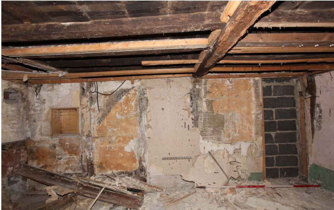
Illus. 19. The northern gable of the hall showing its largely intact framing with internal arch-braces and two studs flanking the central post which supports the axial ceiling joist. Note the recently blocked door (right) and the serving hatch (left) that formerly linked this room to Pottery House. These features were previously hidden by dry-lining and were probably blocked during the post-1963 restoration.
