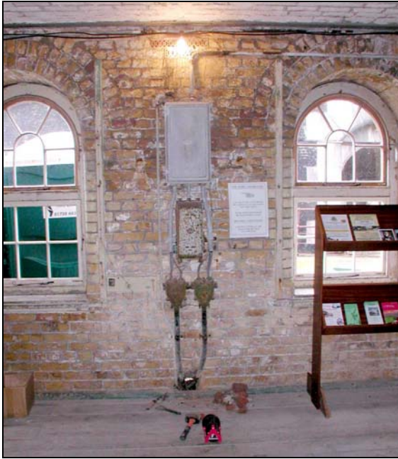
Plate I: View inside Guardroom. The new electrical box is to be fitted in the location of the white notice adjacent the window
