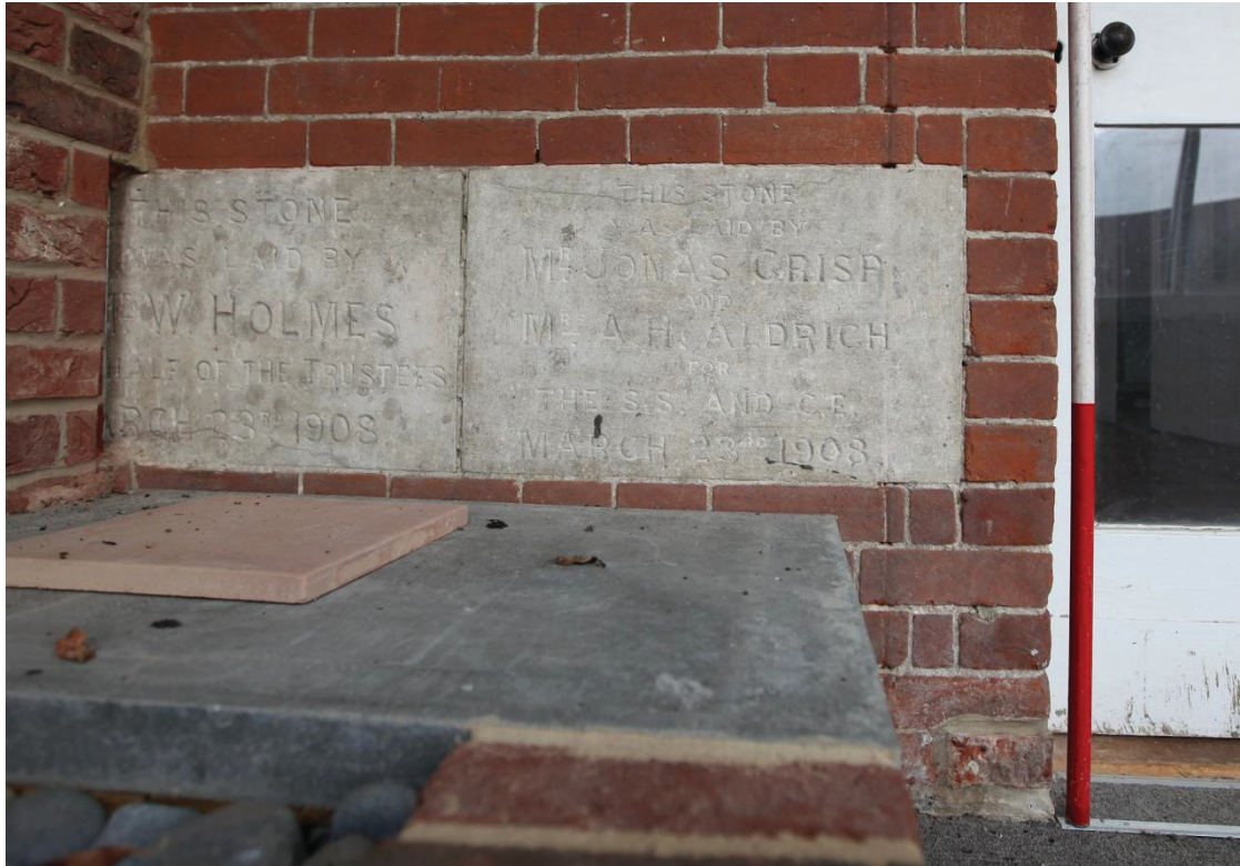
Illus. 7. A detail of the inscribed foundation stones to the north of the external doorway of the 1908 Sunday School wing (3). THIS STONE WAS LAID BY MR W. HOLMES ON BEHALF OF THE TRUSTEES MARCH 23rd 1908 (left); THIS STONE WAS LAID BY MR JONAS CRISP AND MRS A.H. ALDRICH FOR THE SS AND CE MARCH 23rd 1908 (right).
