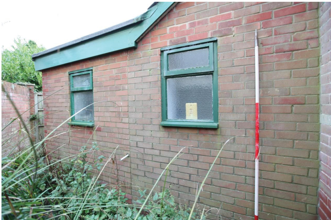
Illus. 12. The northern exterior of the late-20 th century lean-to WC extension (4) with the eastern gable of the Sunday School (3) on the right and the additional flat-roofed extension (5) which forms a rear lobby on the left. The site is closely confined by the property boundaries of the adjoining 20 th century houses.
