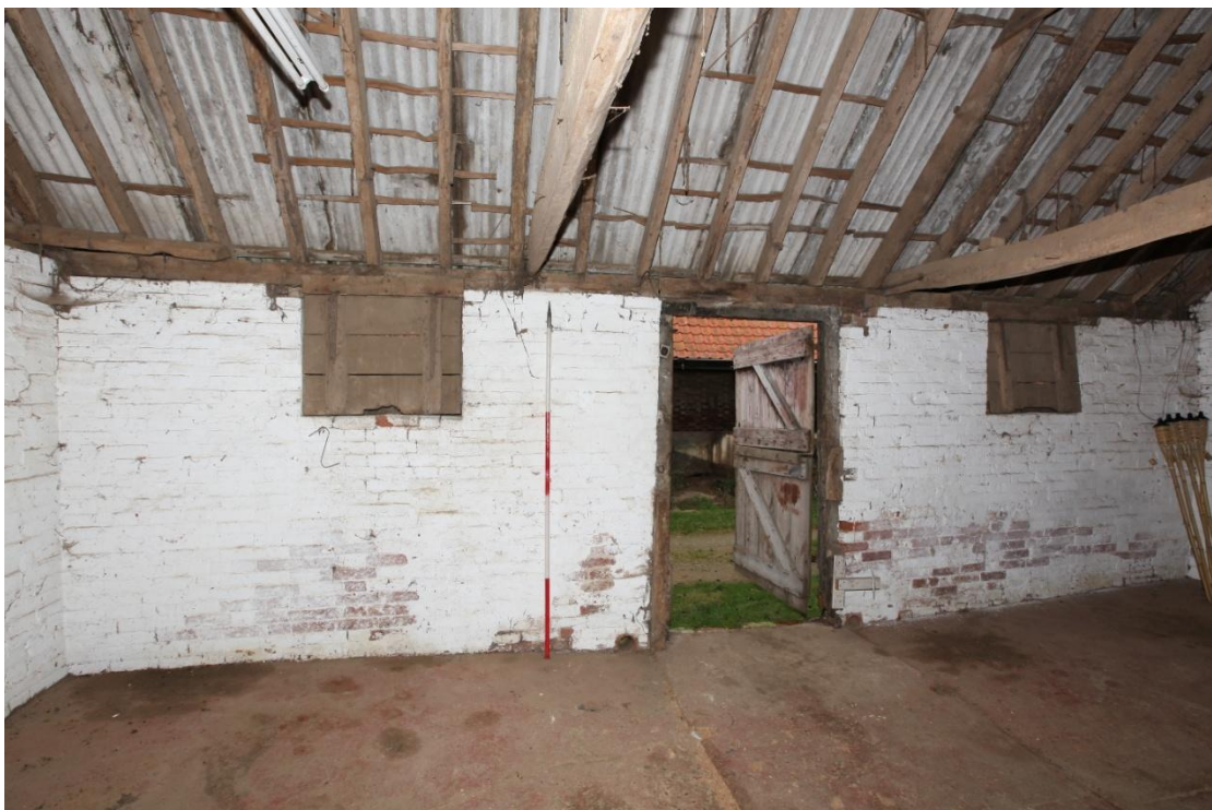
Illus. 10. The northern interior of the 19 th century stable (4) showing its original central entrance flanked by vertically hinged shuttered windows with floor drains.
