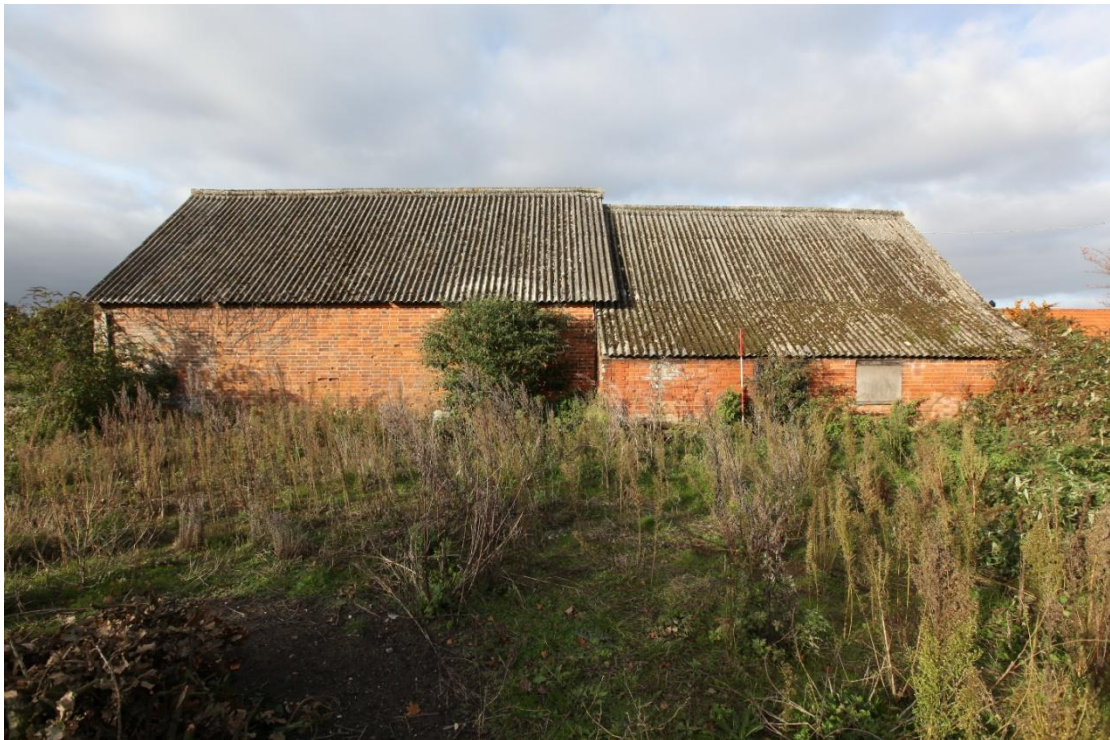
Illus. 6. The rear (southern) exteriors of the cart lodge (3) to the left and the mid-19 th century stable (4) with its integral lean-to on the right. Both roofs are clad in 20 th century corrugated asbestos.
