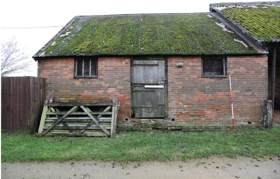
Illus. 8. The northern facade of the original 19 th century stable (4) showing its central half-hung door flanked by shuttered windows - all respected by closer bricks. Note the circular drain apertures marking the internal floor level.
