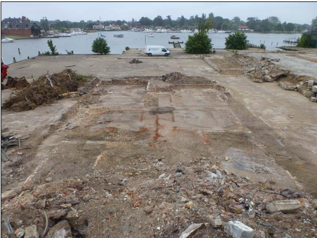
Plate 6. Area of Trench 3 (prior to excavation), showing wall lines of former 19th century structures, camera facing south (ref. HWZ 73)
