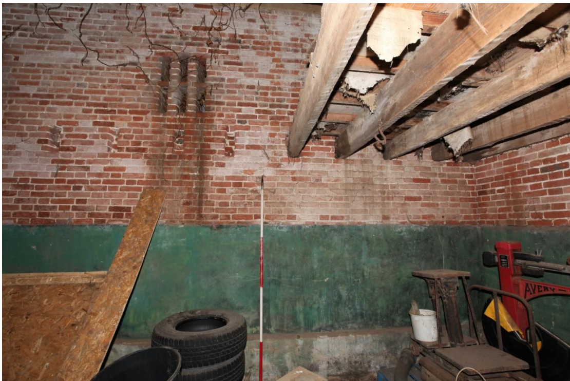
Illus. 10. The western end of the southern interior showing the remnant of a late-19 th century loft adjoining the western gable on the right. A series of crudely cut apertures for missing joists can be seen in both the front and rear walls of the entire western half of the barn. A new floor of 20 th century axial softwood joists is visible above the 19 th century lateral joists.
