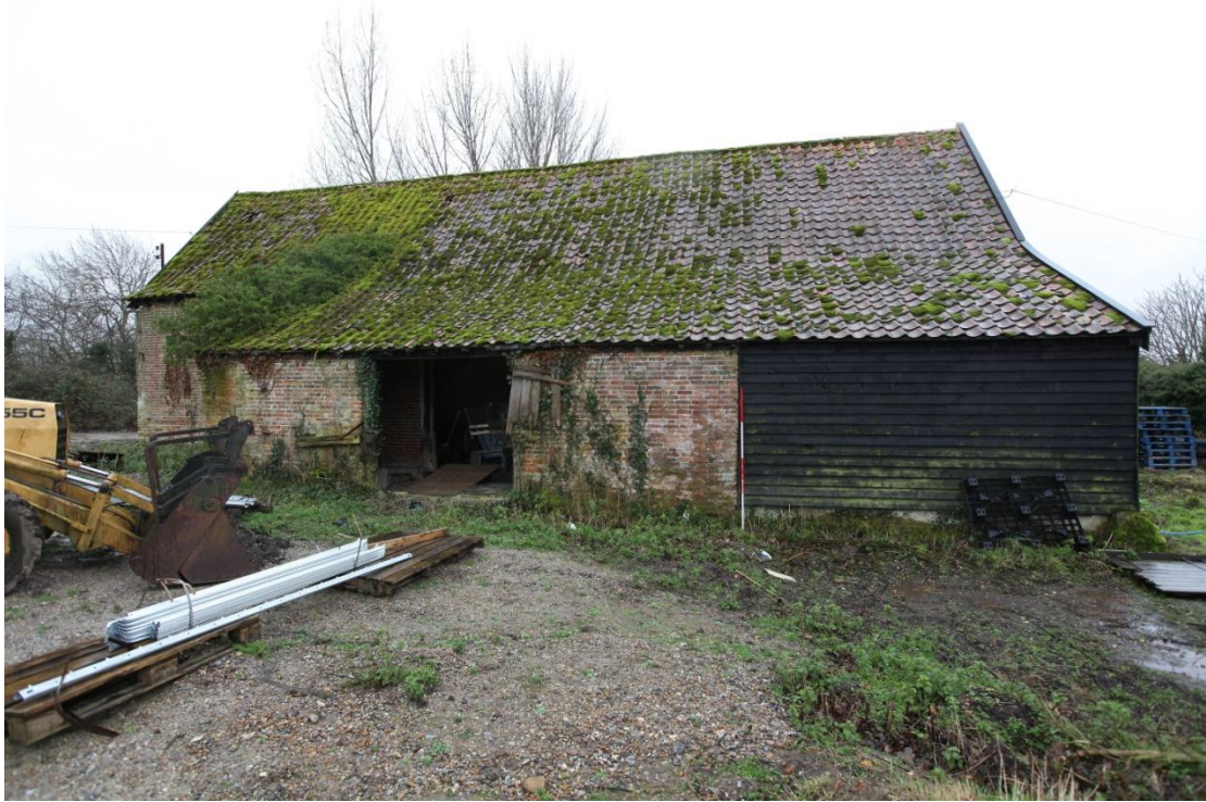
Illus. 3. The rear (northern) exterior showing the central lean-to brick porch added in the mid-19 th century to increase the length of the threshing floor and provide grain storage bins on each side. The weatherboarded studwork to the right was renewed in the 20 th century.
