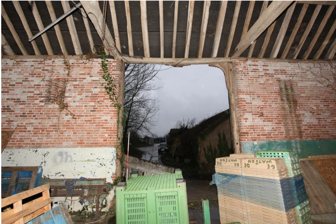
Illus. 9. The southern entrance flanked by ventilation loops arranged in groups of three over three. The right-hand (western) door jamb and bolted knee-brace appear to be original, but the left-hand jamb is a replacement and its knee-brace has been removed. There is no evidence of a threshing floor but it may survive beneath modern concrete.
