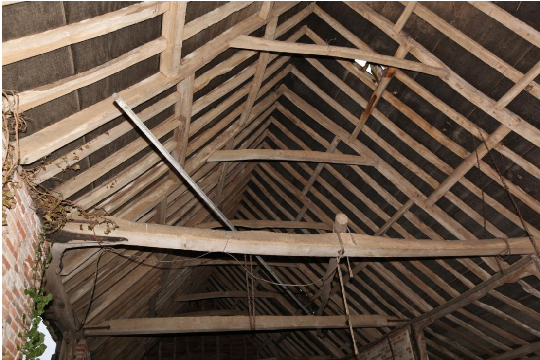
Illus. 7. The intact, original oak roof structure consisting of two tiers of staggered butt-purlins with pegged collars. This form of roof is typical of the late-18 th and early-19 th centuries in Suffolk.
