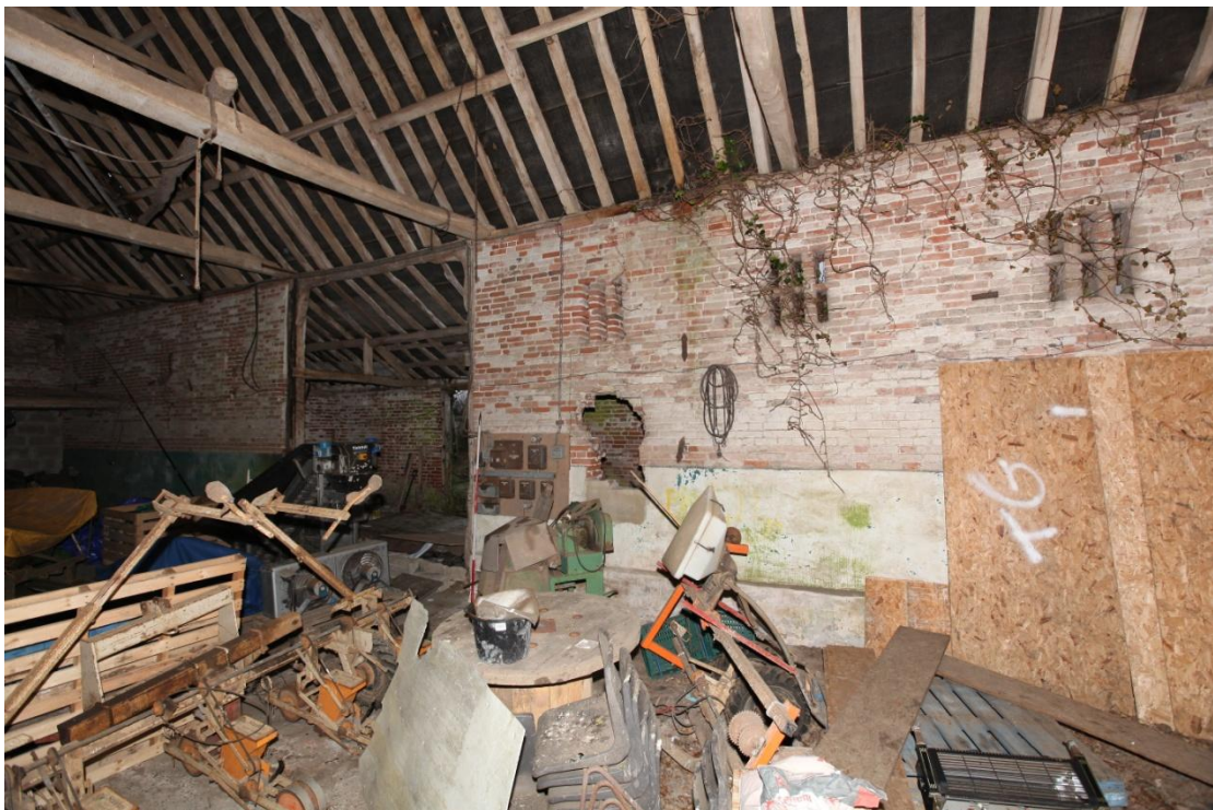
Illus. 6. The northern (rear) interior of the original threshing barn showing the secondary central aperture adjoining the rear porch with three groups of ventilation loops on each side. A hole has been cut through the wall to the right of the porch in recent years, perhaps to accommodate a drive shaft.
