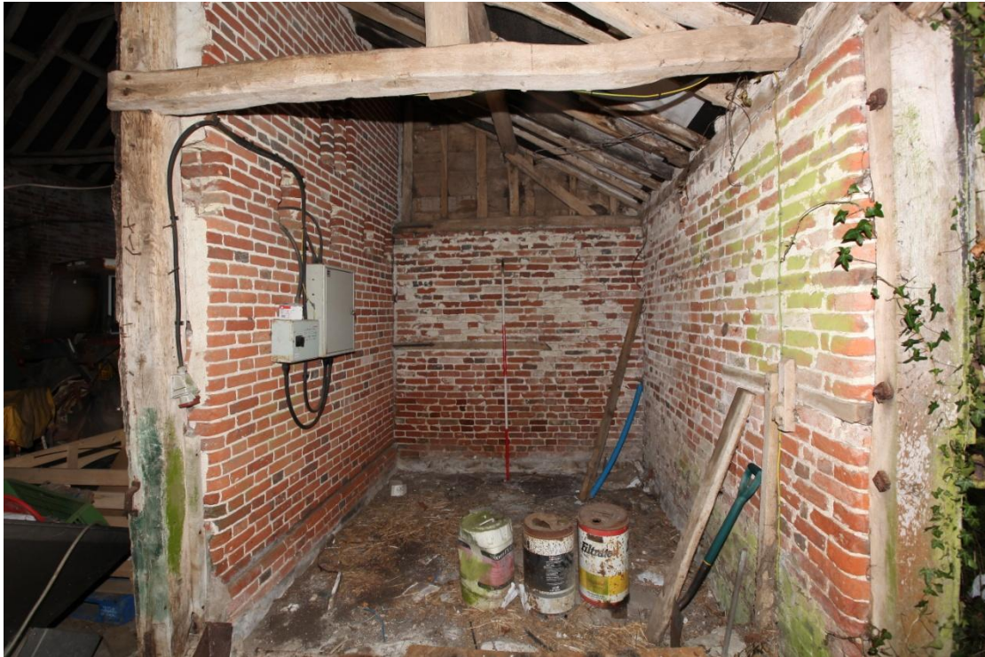
Illus. 5. The western half of the secondary lean-to rear porch, with the grooved wooden post of a grain bin still attached to the northern wall on the right. The entrance to the barn on the left has been cut through the brickwork and is secondary, having replaced a smaller original back door.
