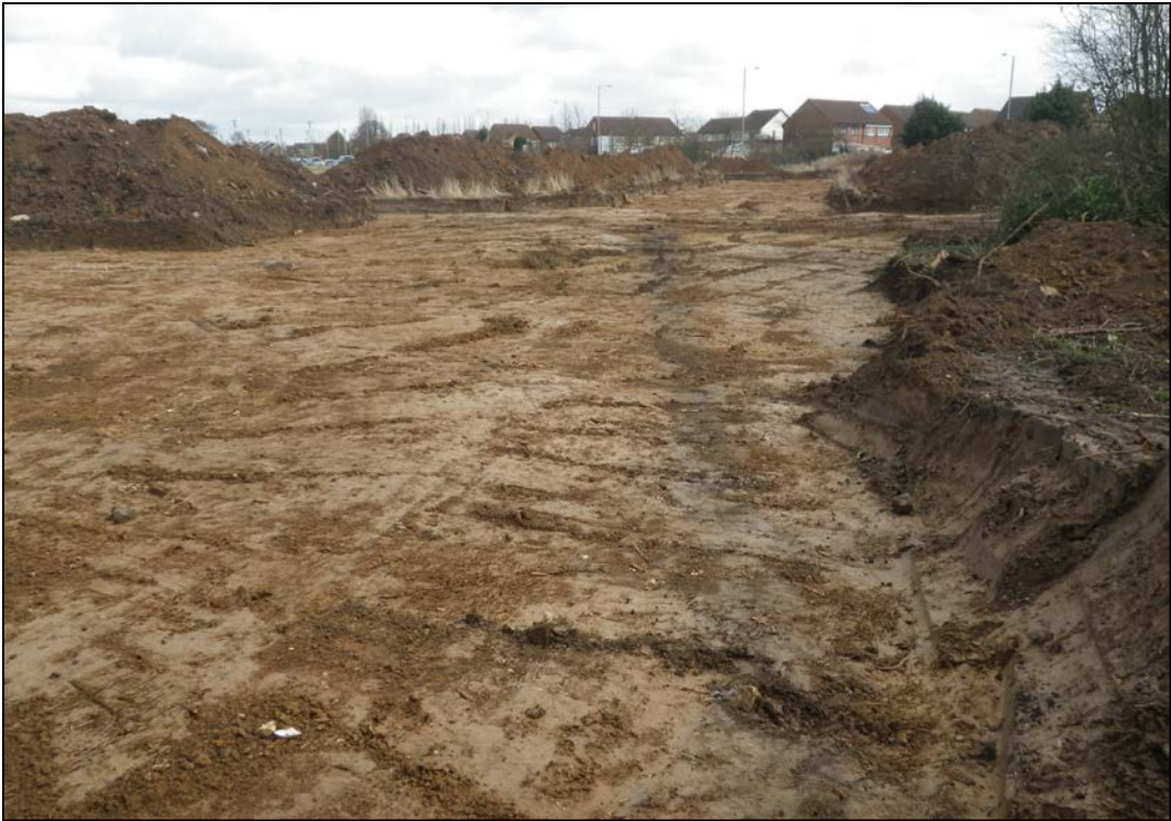
Plate 1. Ditch 0007 (centre right) visible running across the excavation area camera facing south (ref. HWX65)
