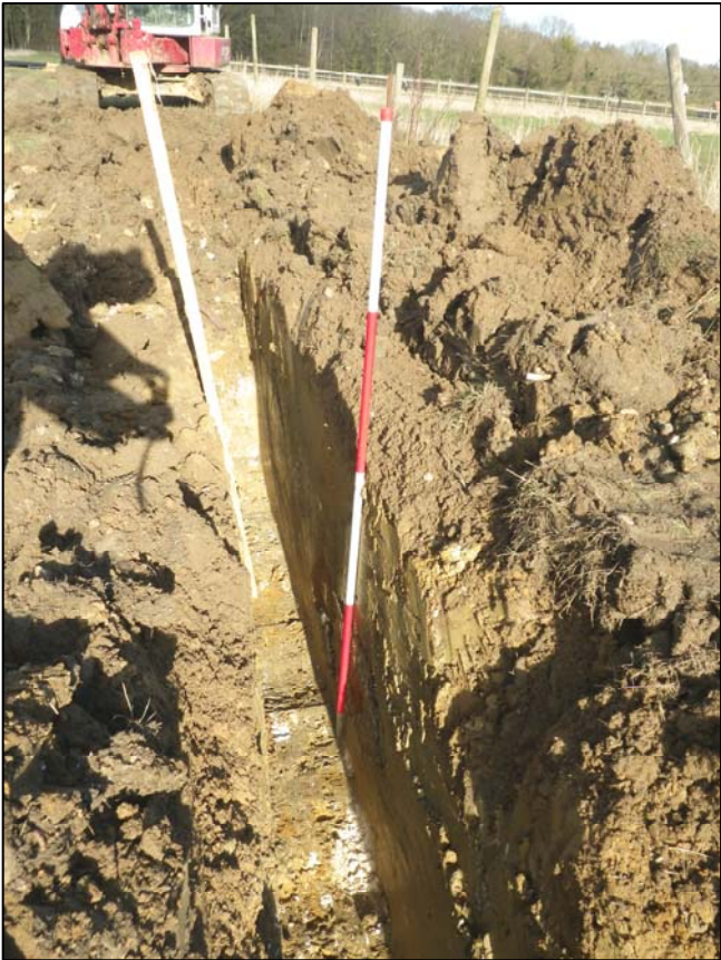
Plate 2. general view of cable trench at location 7 in Fig. 2, camera facing northeast (ref. HWU 84)
