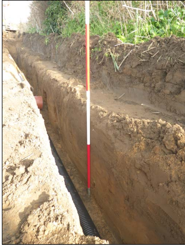
Plate 3. general view of cable trench at location 10 in Fig. 2, camera facing east (ref. HWU 85)
