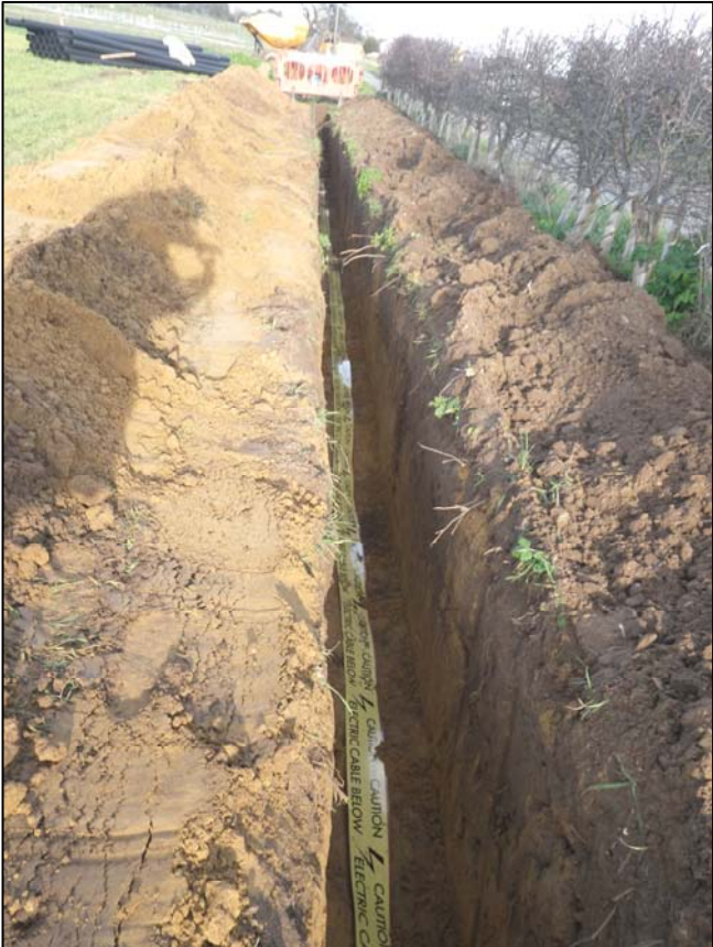
Plate 1. general view of cable trench at location 2 in Fig. 2, camera facing east (ref. HWU 83)
