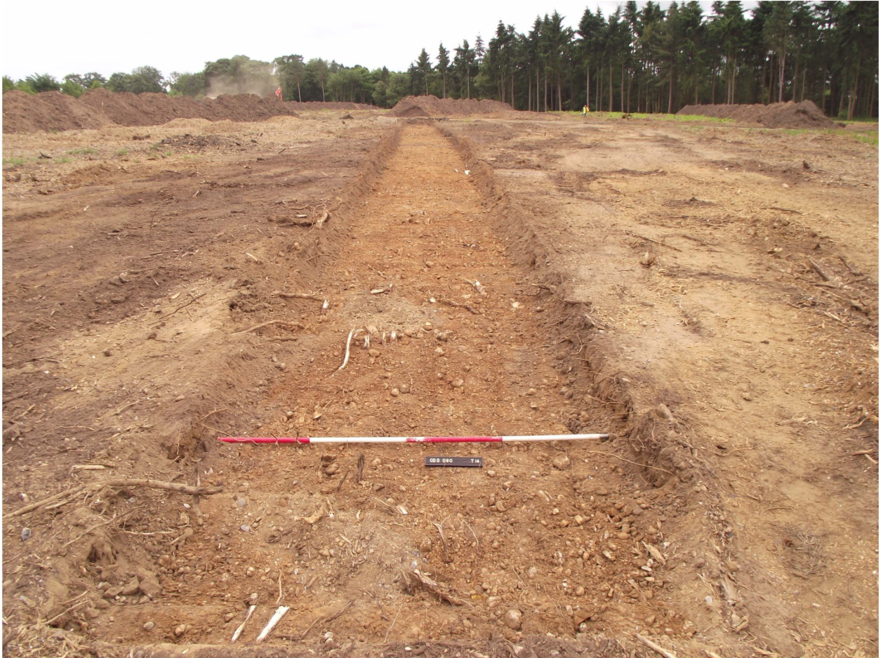
Plate 1. View of Trench 14 looking south; note shallow depth of trench and degree of tree root disturbance across base of trench. Beyond the trench large 'windrows' can be seen which contain material from the mulched tree stumps and scrape across the topsoil.
