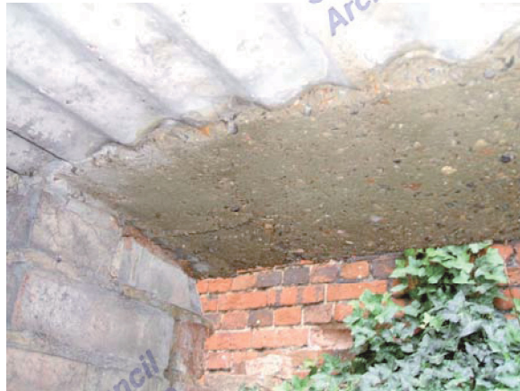
Figure 6. Inside of the roof at entrance showing limit of corrugated iron impressions
