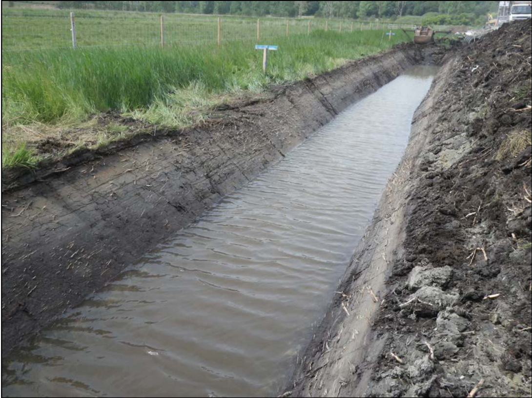
Plate 7. Realigned ditch at toe of western flood bank, camera facing northwest (ref. HWS 42)
