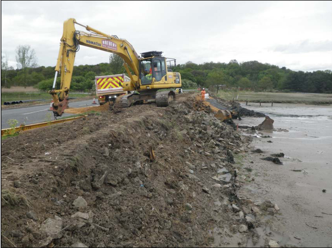
Plate 5. east face of causeway after removal of rock armour, camera facing north (ref. HWS 42)
