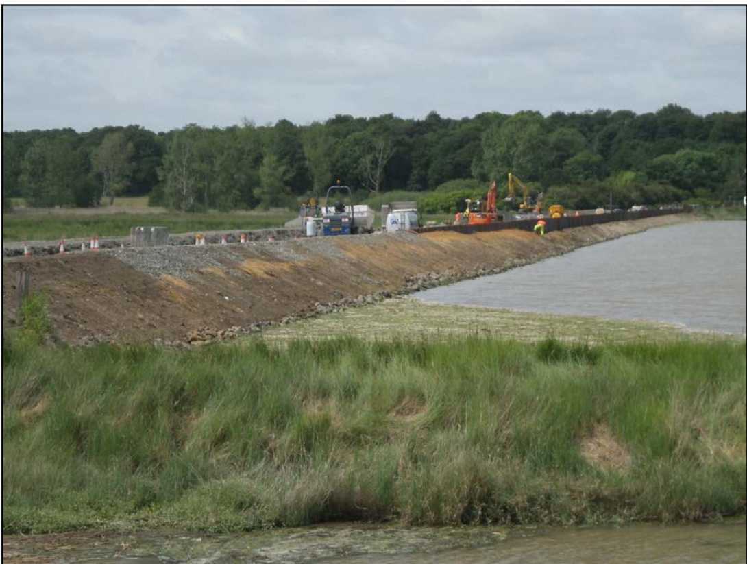
Plate 8. East face of causeway after insertion of sheet piling, camera facing northwest (ref. HWS 66)
