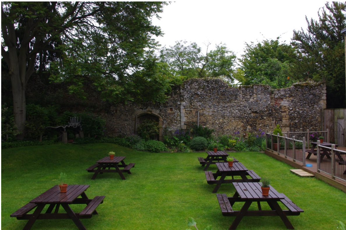
Plate 3. The surveyed door alongside the end gable of Building 1 (which extends to the wooden fence at the right of the picture). Soil imported in the 17th century buried the bottom of the ruins; the level in the refectory garden has since been reduced (note ground surface below the tree to the left) but the level of the picnic lawn is still c.120mm above the medieval threshold level. The floor of the building was sunken below this and was not found during the current work.
