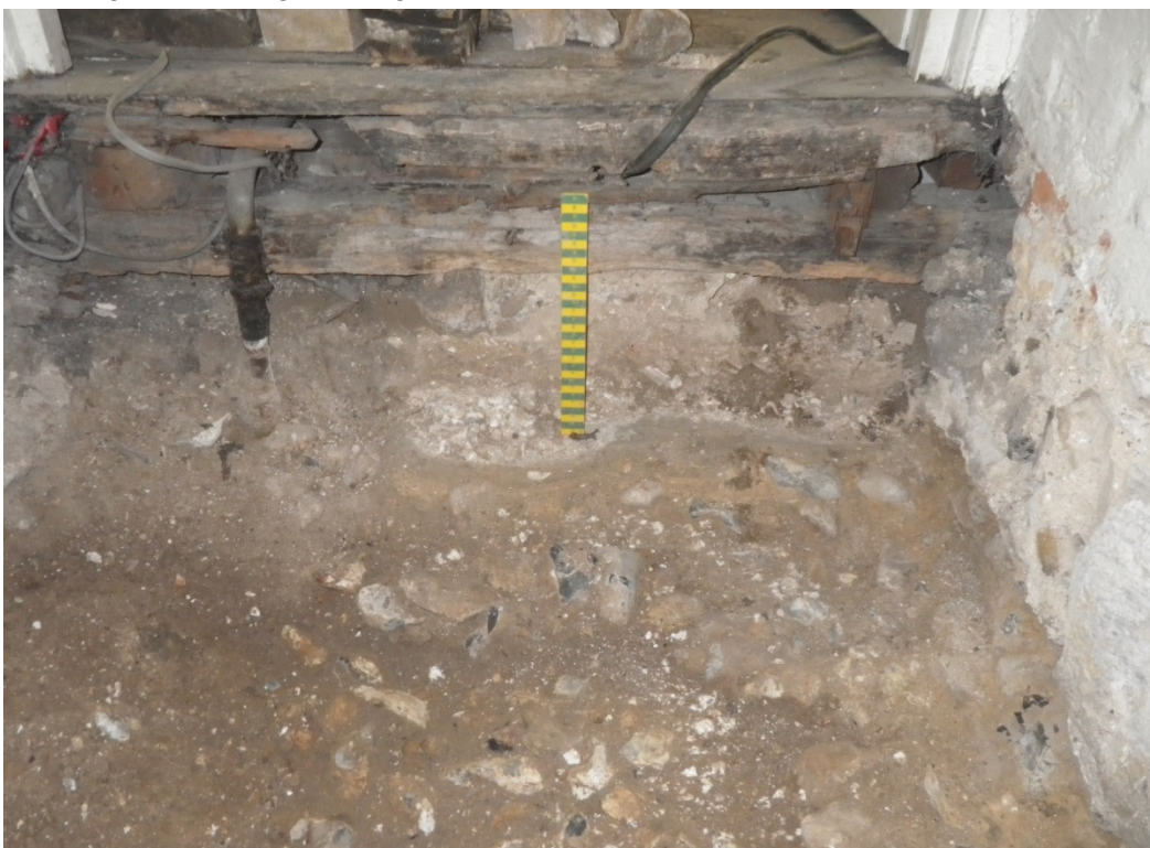
Plate 10. Test hole 7 showing the remains of the riser, for the step up to the suspended floor in the Guildhall lobby attached to the end of the floor joists. The timber floor was laid over a previous chalk floor (behind the scale) which partially covered the truncated rear wall. Of the rear wall, only a single course of bonded flint work survived where the door opening appears to have been lowered and the flints at the bottom of the picture are the packing of the foundation trench seen in plan.
