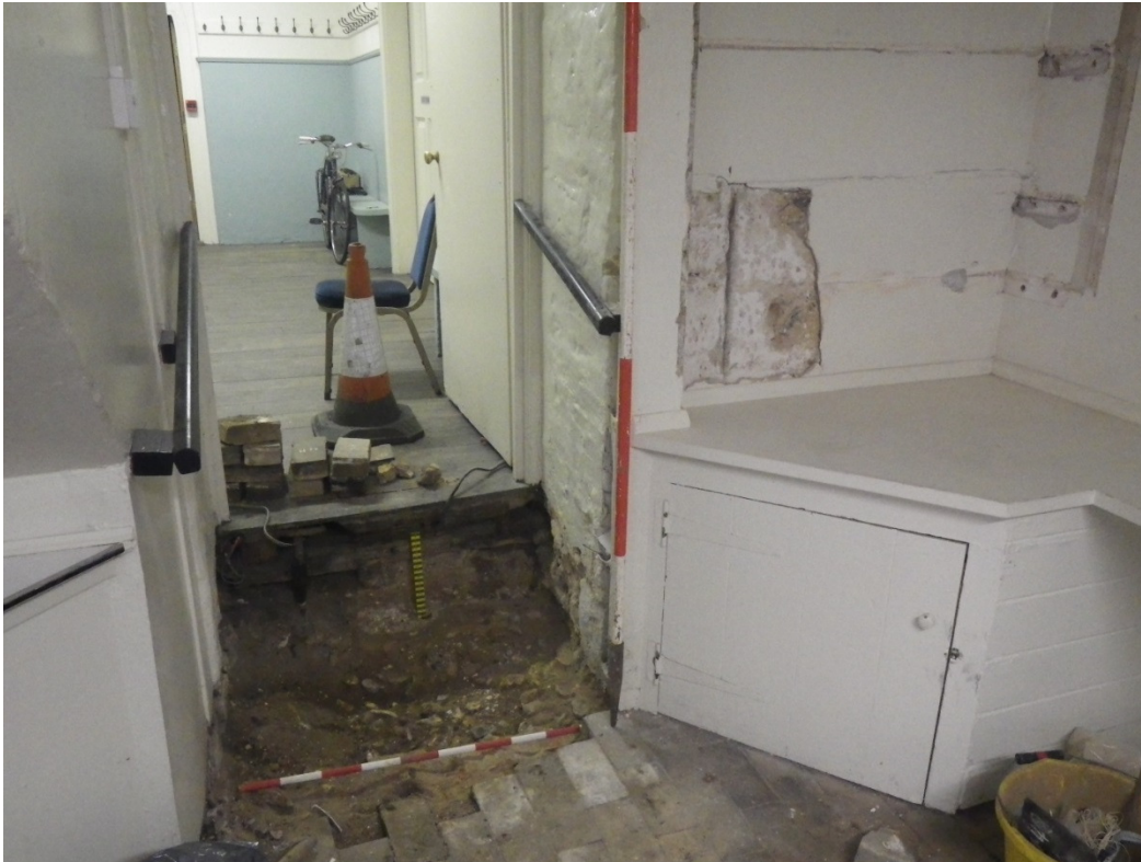
Plate 9. Test hole 7 in the doorway between the medieval Guildhall and the early 19th century kitchen. The doorway was reduced in width during the 18th century and the edge of an earlier opening, with limestone dressings, can be seen where the plaster was removed to the right of the door. The door threshold appears to have been lowered to match the brick-paved floor of the rear range truncating the original threshold and wall. The scale is marked in 0.5m divisions
