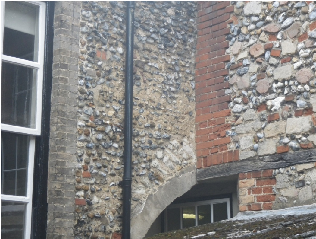
Plate 11. The top of the arch-headed opening over the central doorway through the Guildhall rear wall. The stone dressings of the arch soffit appear to have been removed and replaced with brick/tile rendered over with cement (see plate below). The strainer-course over the arch of pale-coloured clunch fragments is original and fits with the flintwork of the rear wall without interrupting the coursing; clunch is also incorporated amongst the horizontally coursed flint to the left of the arch demonstrating that this material was being used as part of the general build. The plans of the Guildhall suggest that the arch spanned two doors and the half shown in the picture gave access to a covered passage (now removed) to the detached kitchen (see Fig. 7).
