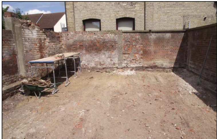
Plate 1. Site as seen on 12th June after removal of the existing concrete slab
