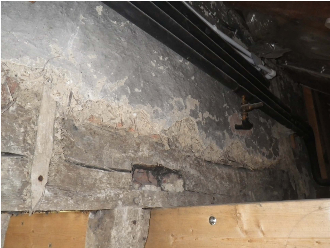
Plate 8. Rear wall of the kitchen, formerly the exterior wall just above the mid-rail. The infill between the studs was brick rubble behind split lathes nailed to the frame and rendered with a course daub; this treatment of the wall post-dates the style of the 16th century work seen at the eastern end of the building suggesting extensive reworking of the building in the 19th century.
