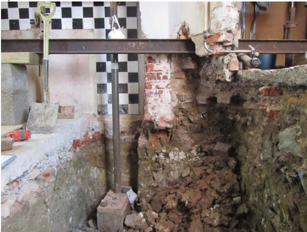
Plate 4. The large fireplace may have been reduced in width in the 18th century with the addition of the slender pier in the centre of the picture. The south (exterior face) of the chimney was subsequently altered in the 19th century with the addition of a (?) bread oven or a copper, the floor of which was preserved 300mm below the current concrete floor. The construction of the bread oven /copper necessitated the removal of a section of rear wall and was accessed from a lean-to rear range which was added to the back of the building in the 19th century.
