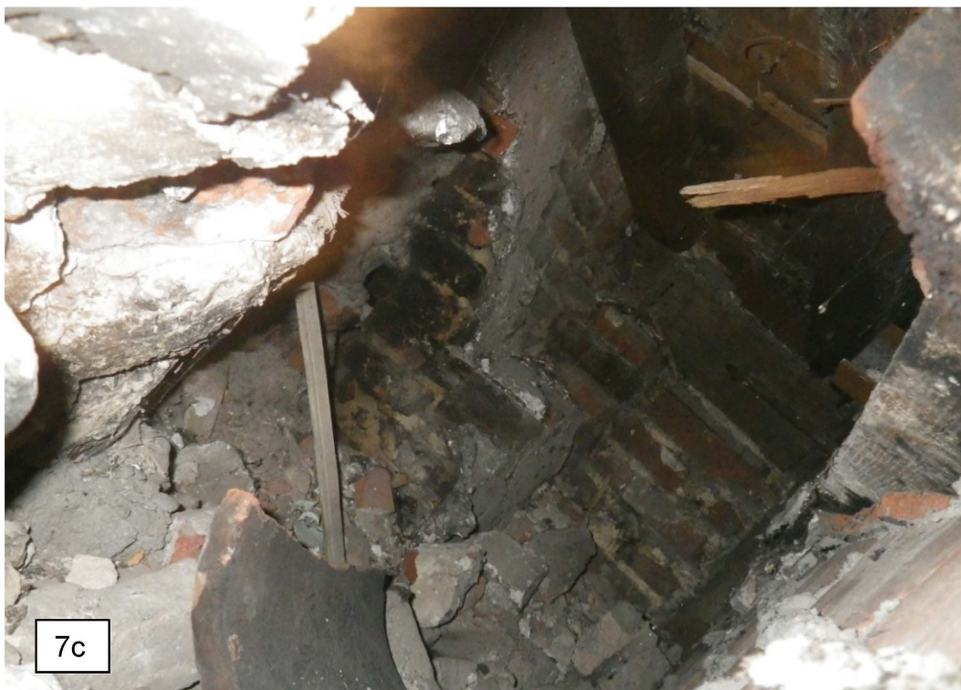
Plates 7a) b) and c) The removal of the brick-built section of the kitchen's back wall revealed a complicated void between the wall and the south pier of the chimney. Previously this space had included a possible bread oven; the sooted interior of which can be seen top left. The bread oven was a late addition which breaches the line of the original rear wall and necessitated the removal of the studs from the lower wall along with the lower half of one of the principal posts. The empty stud mortises can be seen in the underside of the mid-rail (top right) which also included the setting for two small single-bar mullion windows. The unlikely juxtaposition of a window to the fireplace suggests that either the fireplace is inserted or that the timber is reused. The bottom image shows the shoulder of the original fireplace with the cross beam on the east side of the chimney tied to back wall with an iron strap rather than jointed
