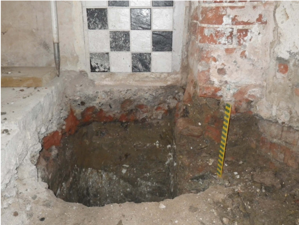
Plate 5. Excavations within the fireplace alongside the south pier, showing a layer of decayed brick, part of a previous hearth predating the existing fireplace. The extent of the hearth continued beneath the existing fireplace pier and the two were separated by an intervening layer of green boulder clay. Charcoal residue was observed over the brick hearth and beneath it was sealed a thin layer of charcoal and disturbed clay evidence of an occupation of the site that predated the existing house.
