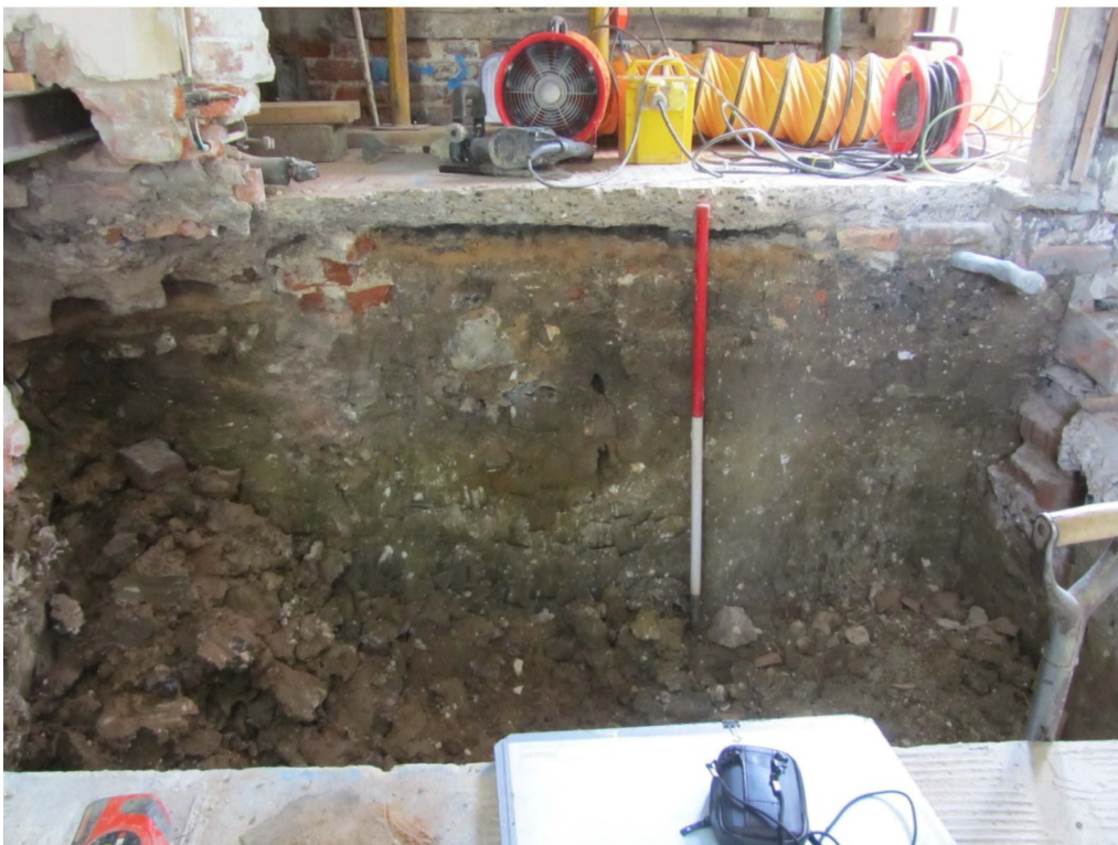
Plate 6. The soil profile beneath the floor of the rear range after the back wall of the kitchen had been removed. The concrete was laid over a brick parget floor beneath which was a 500mm depth of disturbed soil which contained brick and mortar rubble, charcoal throughout and mortared flint. The top of the undisturbed boulder clay (at the division in the scale) was riven with a v-shaped, silt-filled feature.
