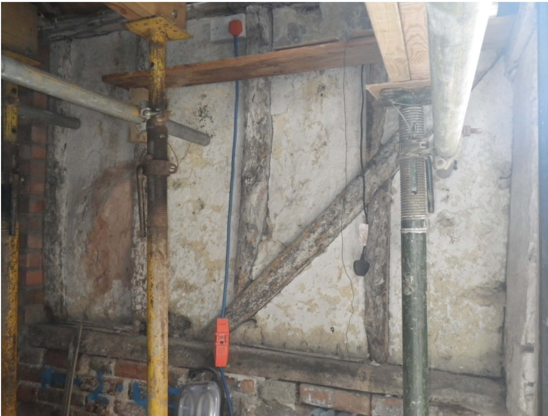
Plate 9. The timber-framed wall of the rear extension with interrupted studs indicative of 19th century framing
