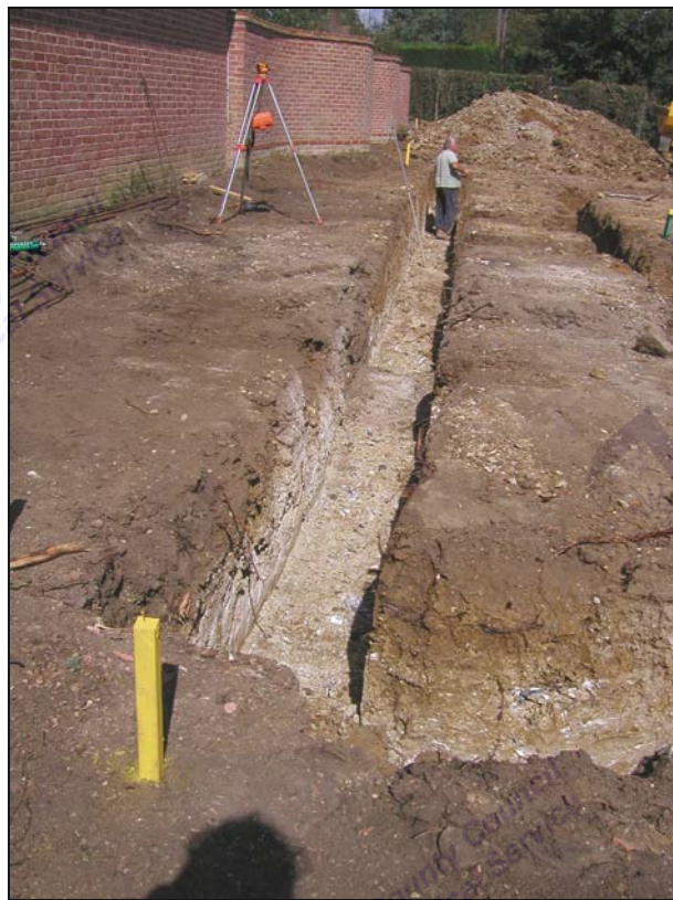
Plate I: Footing for the western wall of house. The brick lined structure is visible in the centre of the picture
