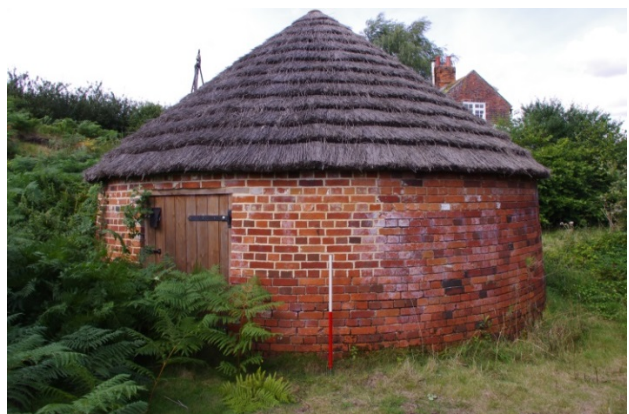
Plate 3. View of kiln looking west, showing rear single door and area of recent repointing
