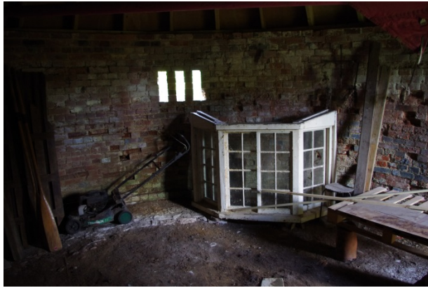
Plate 4. Internal view looking south-west showing slit window and partial floor of white bricks
