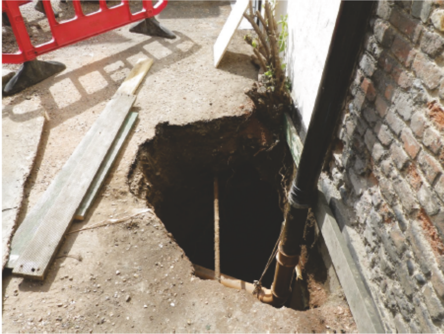
Plate 4. Exploratory hole beneath the downpipe alongside Abbey House revealing the extent of the damage.
