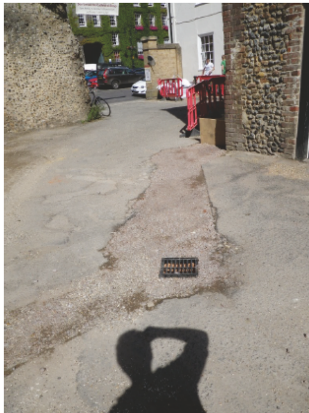
Plate 6. Repaired drain line. No undisturbed layers were uncovered during this work or during the re-laying of the tarmac.
