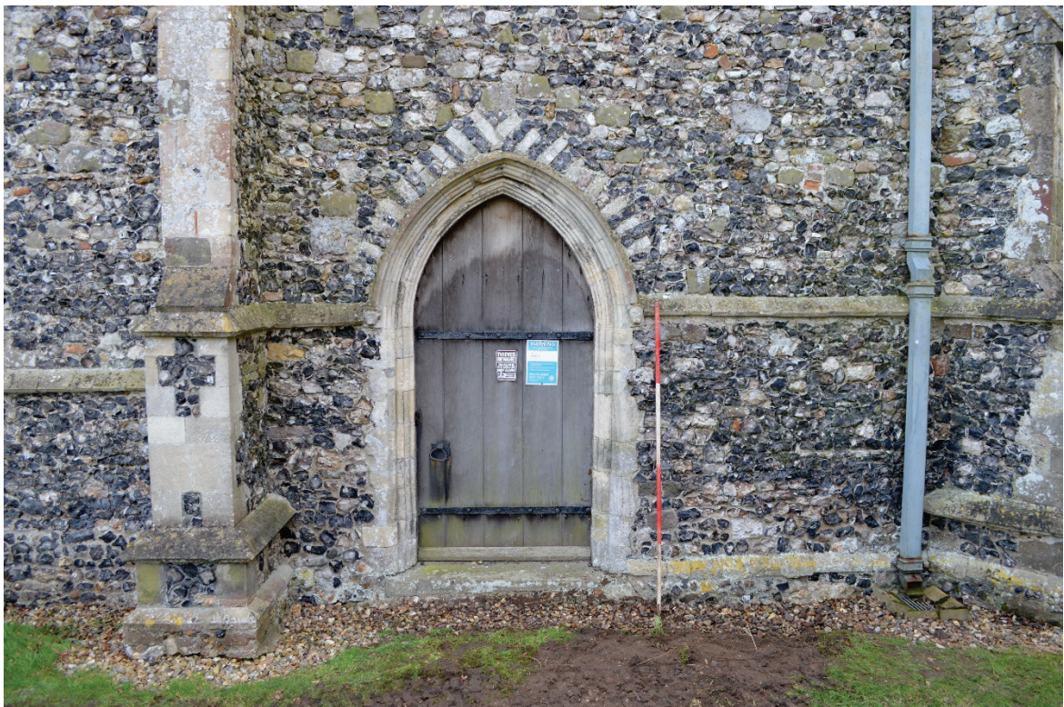
Plate 2. The north door is original to the 15th century aisle and was restored during the 19th century. The new building will extend from and incorporate the buttress on the right and the finished floor level will approximate the existing threshold step.
