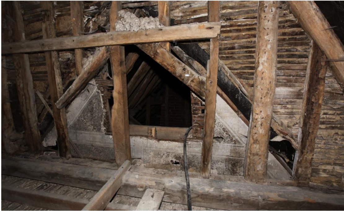
Illus. 5. The plastered and pargeted apex of the original external southern gable of the ‘Cottage’ (4af) seen from the slightly later roof of the brick ‘infill’ (5f) between this and the external southern gable of the 17 th century structure. The pargeting is divided into triangular panels textured with fragments of flint. This gable is weatherboarded at lower levels but the height of the change is unclear.
