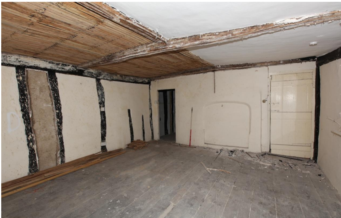
Illus. 8. The chamber over the southern parlour (1af) from the south, showing the outline of a second arched and rendered first-floor fireplace in the central chimney. There is no evidence of windows in the rear wall to the left. As elsewhere in the house the roof-plates and ceiling joists were all rendered originally, with large split oak laths nailed to their surfaces, but this render has been removed as part of the present work. The ceiling laths to the left are new. Note the wide oak floorboards.
