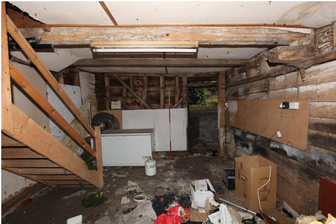
Illus. 4. The interior of the weatherboarded stable (4c) from the rear (west) showing a modern stair to the left and the end of the axial ceiling joist of the adjoining ‘Cottage’ (4b) which projects through the internal partition on the right. The framing of the front wall is typical of the early-19 th century with narrow studs interrupted by nailed diagonal primary braces. The nailed rungs of an original loft ladder are visible to the left.
