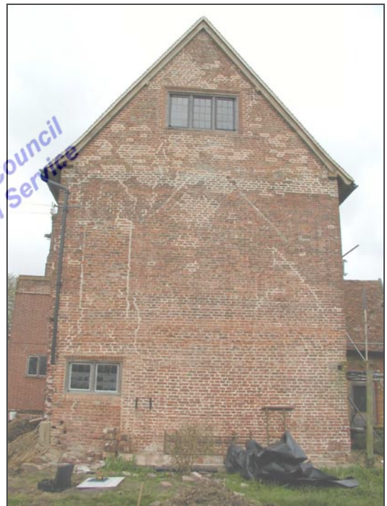
Plate 56 Blocked doorway & gable scar
