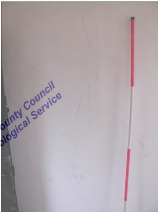
Plate 17 Vertical crack in external render
