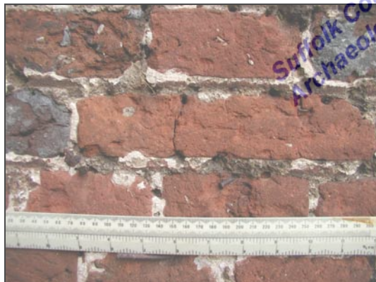
Plate 57 Surviving paint on brickwork
