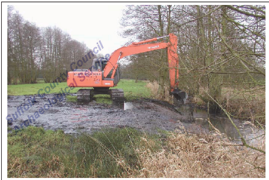
Plate 13: Machining in progress, showing silty deposits removed during reprofiling, Looking south west
