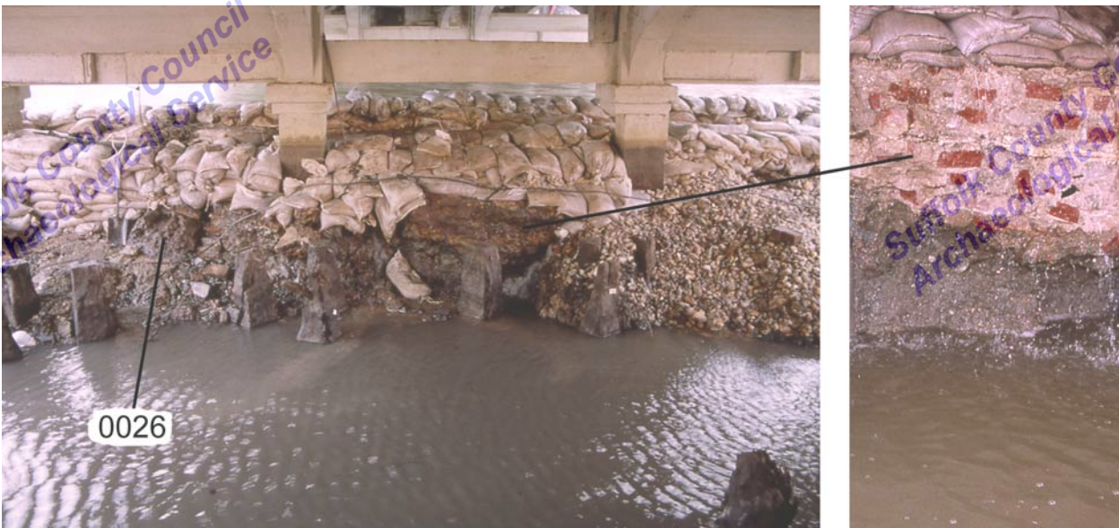
Figure 18. Pier 0025 showing detail of fabric and position of log 0026. In front of 0025 are the timber piles from the later wooden bridge
