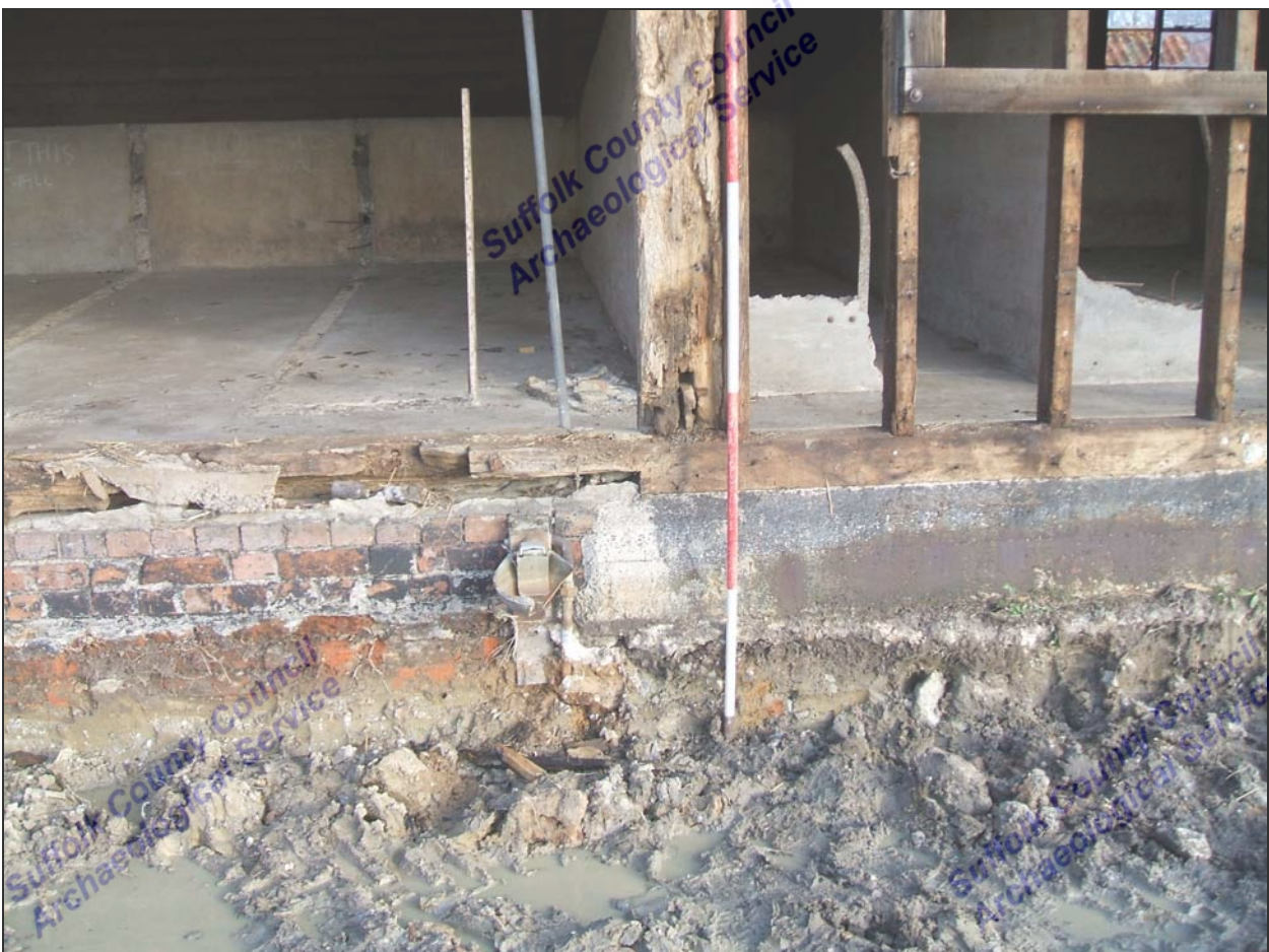
Figure 8. Building 3 West elevation – reused oak post and sill beam at junction of north and central bays
