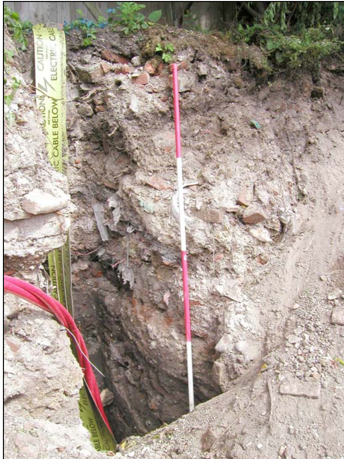
Plate II: Excavation into the slope on northern edge of the site revealing the extensive deposits of made ground
