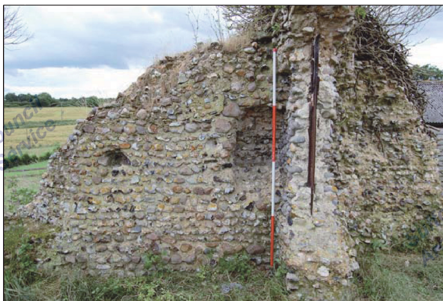
Figure 5. Niche in the chancel south wall also repair to chancel arch using an iron bar.
