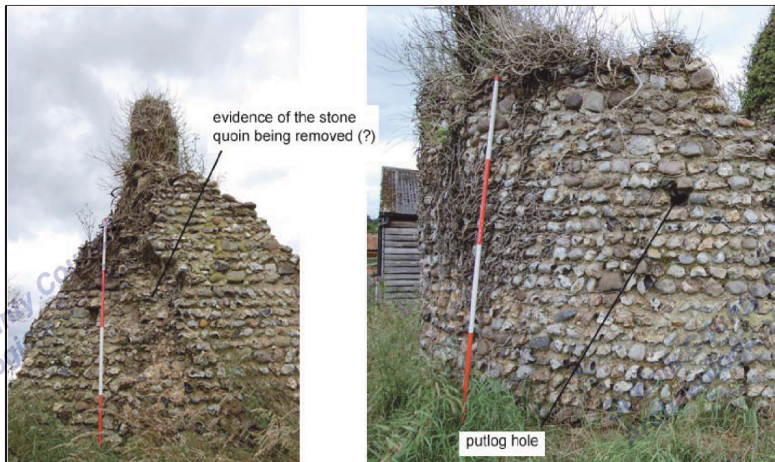
Figure 3. Building details, showing horizontal coursing of the flint, missing quoins and putlog hole
