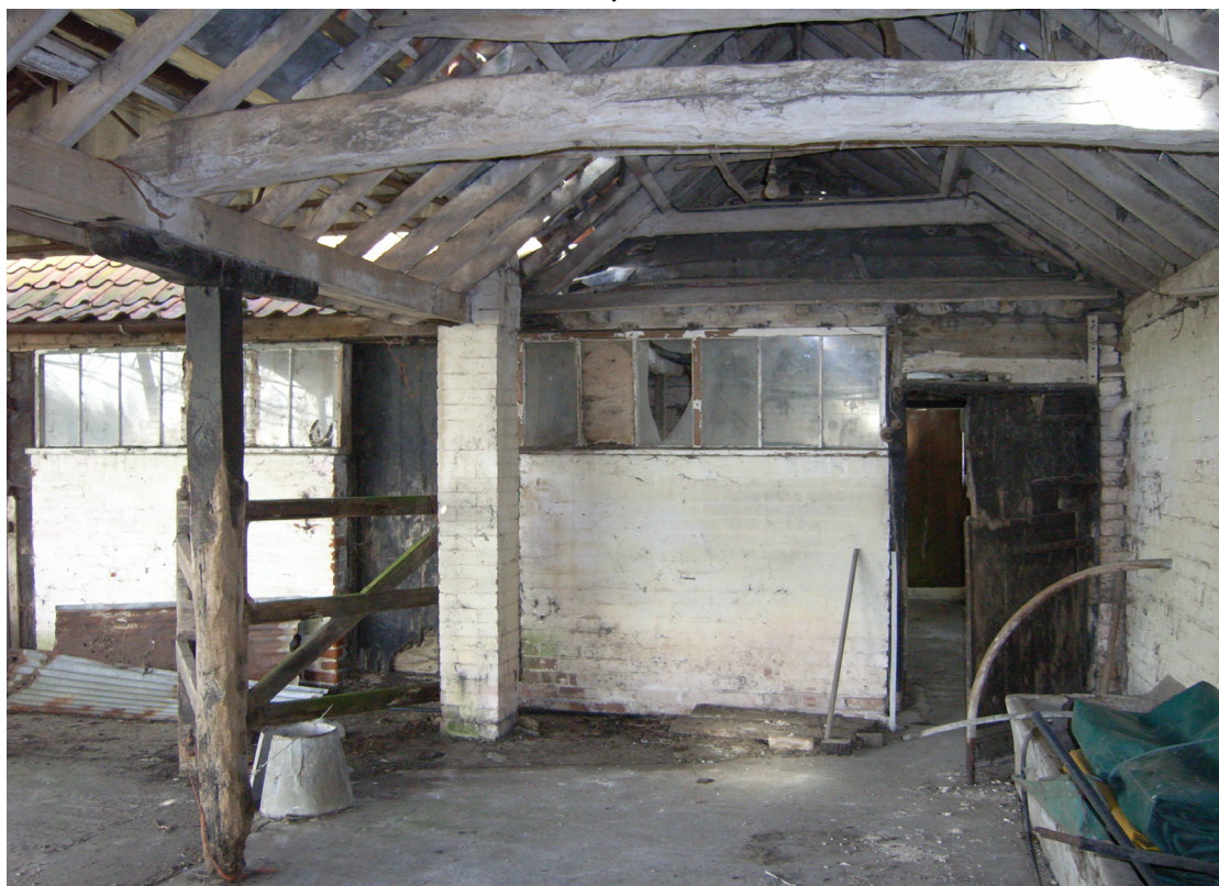
A2.6 Interior of open area (7) in north-eastern corner of covered yard with entrance to shed (4) recently used as milking parlour to right. The gate to left was used to control the passage of cattle. Note concrete trough to right.
