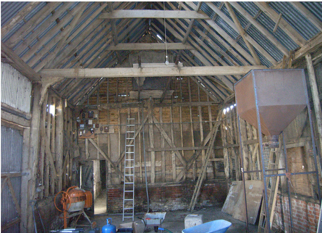
A2.2 Interior of barn from west with inserted door to cattle shed in rear and 20 th century grain hopper to right.
