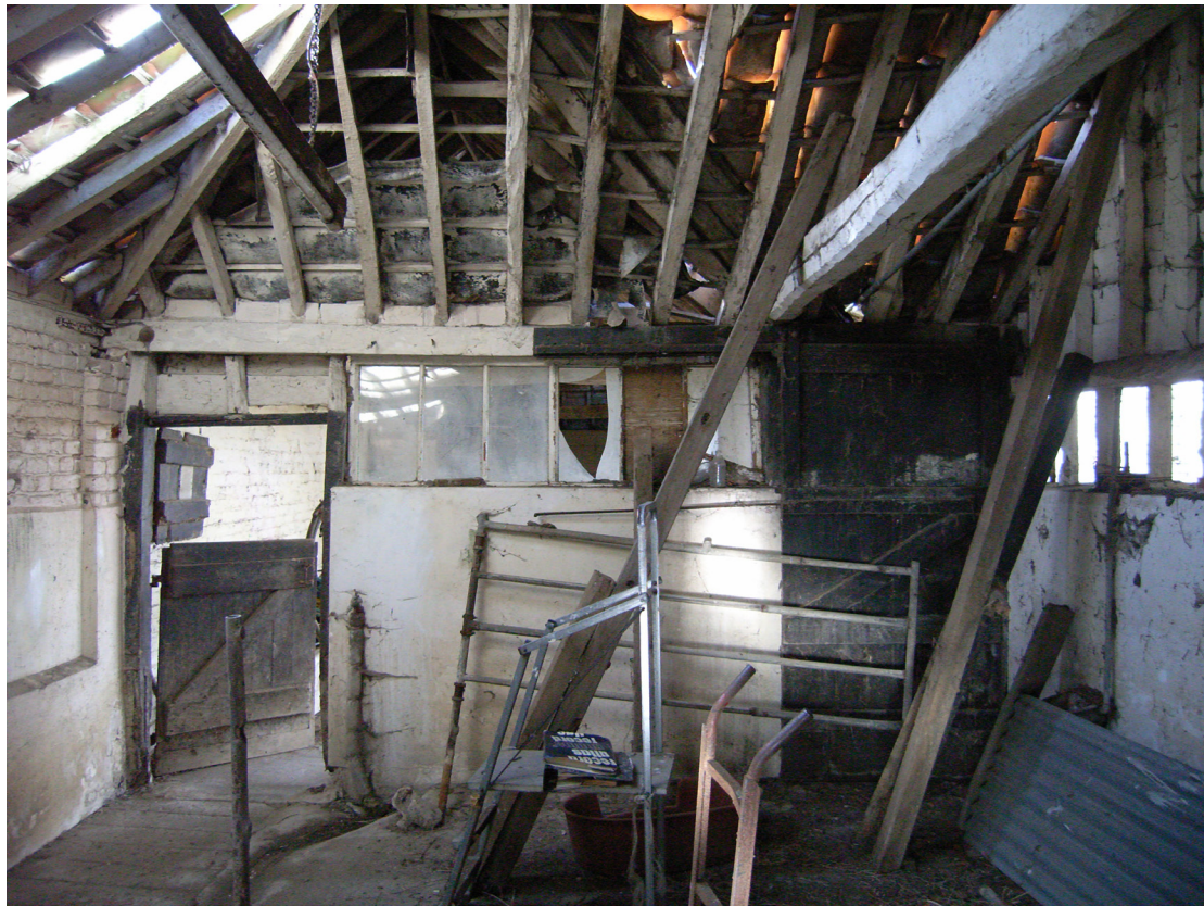
A2.3 Interior of 19 th century shed (4) looking south to open area (7) in corner of covered yard (wall rebuilt in 20 th century). This shed operated until recently as a milking parlour with stalls for four animals facing the wall to the right with floor drain and entrance passage to left.
