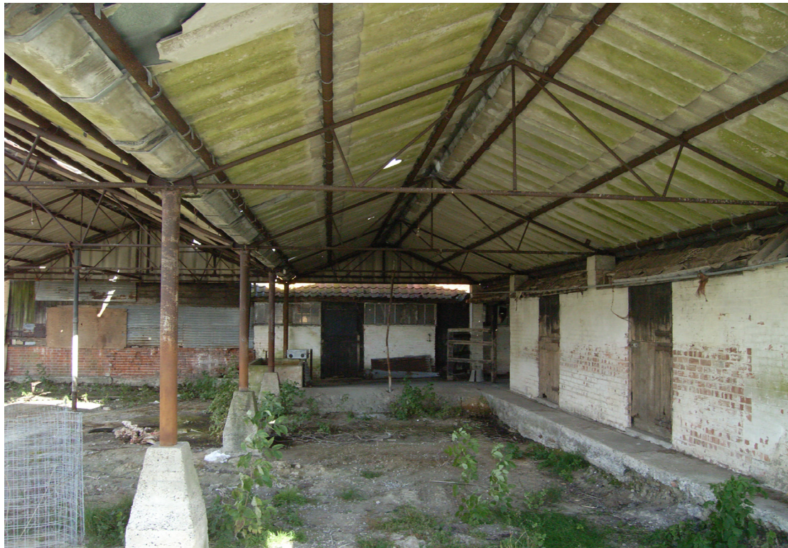
A2.5 Interior of covered cattle yard from the south with mid-19 th century barn and shed in background.
