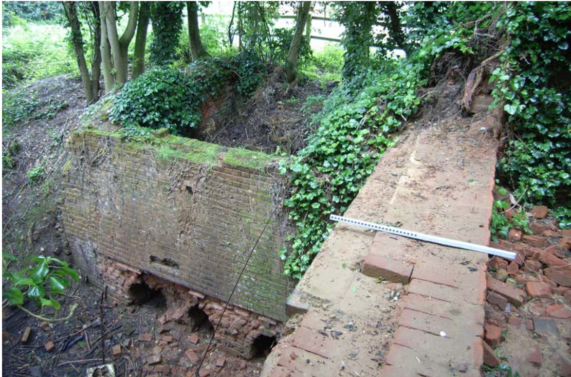
A2.5 The Brick Kiln in the trees shown in A2.1, viewed from the north (the building to be converted lies in background approximately 10 metres away). Included for site context.
