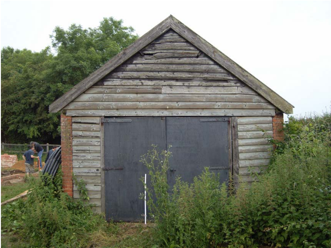
A2.3 External view of southern gable showing replaced double doors to cart shed
