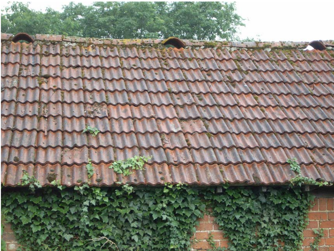
A2.4 Ventilation tiles on the ridge of the stable roof, seen from the road to east.
