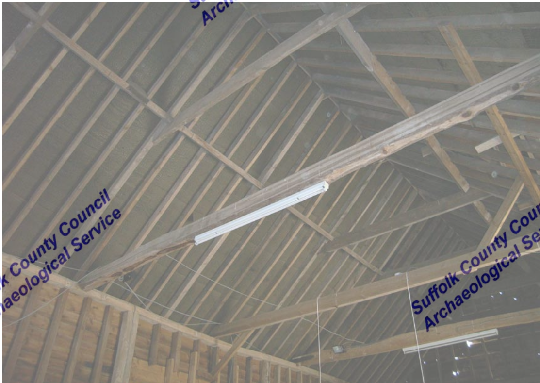
A2.6 Barn B. The original roof structure of the 20 th century barn with its southern gable to the right. The roof has been re-felted.
