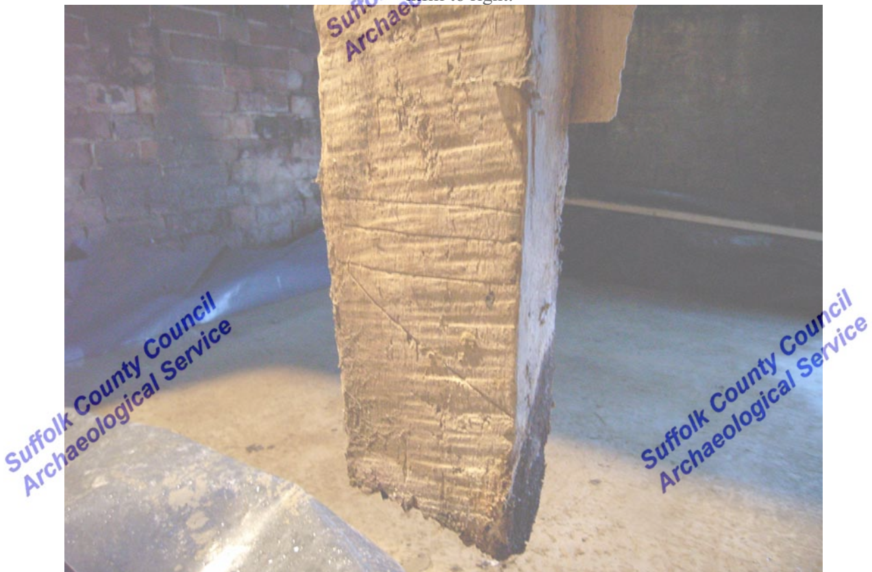
A2.8 Detail of Roman carpenter's numeral to interior base of stud in western bay (no. VII)
