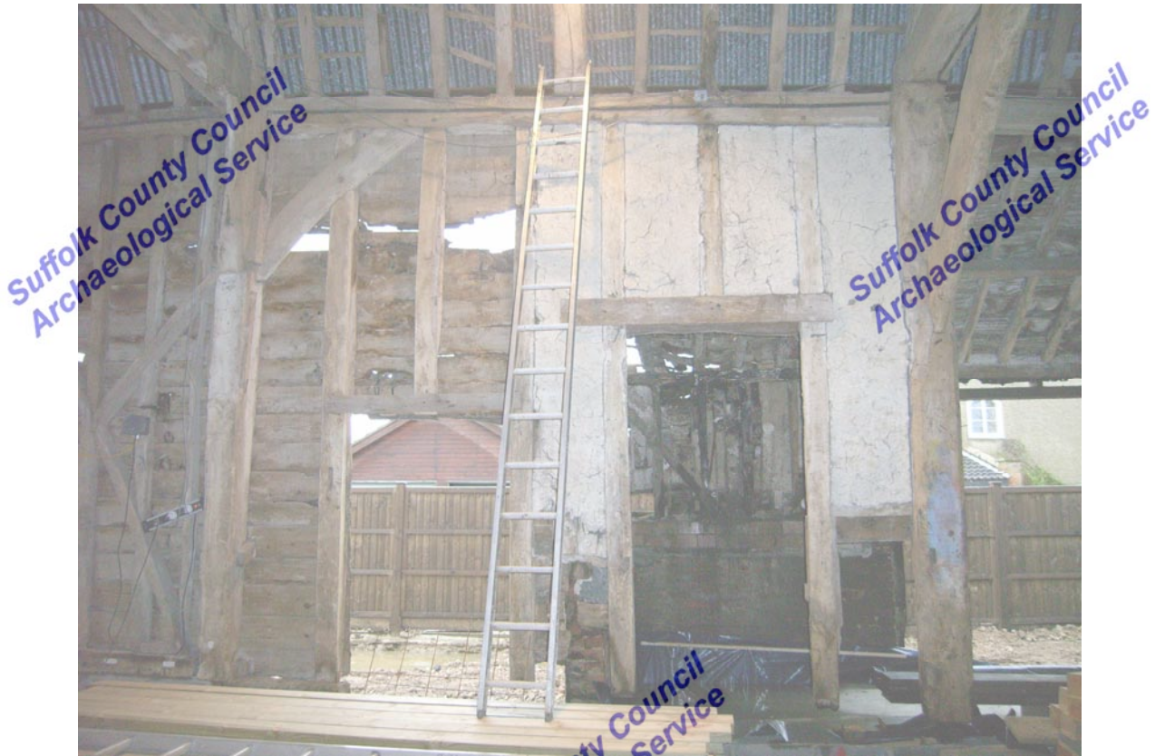
A2.7 Western bay of north-eastern internal elevation showing original wattle-and-daub infill to right.
