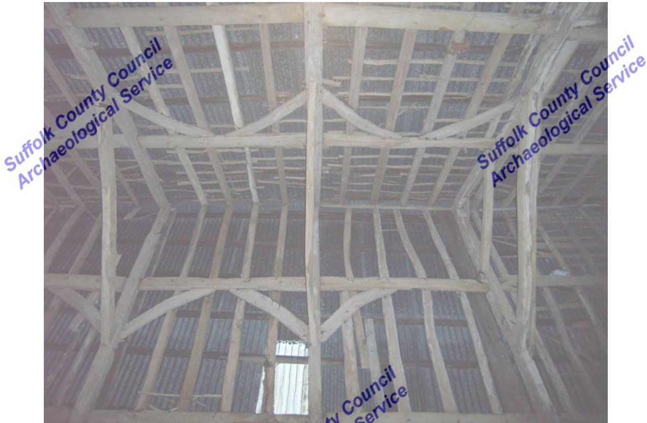
A2.5 roof structure of barn (double butt-purlin with wind braces). Western half showing original north-western gable to right (studwork removed)
