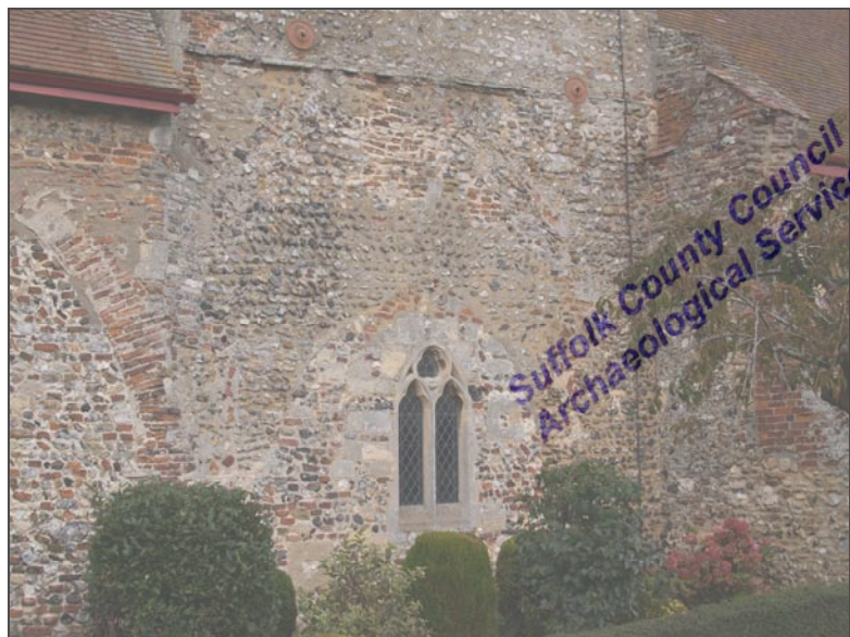
Plate 14 Scar of south transept arch
