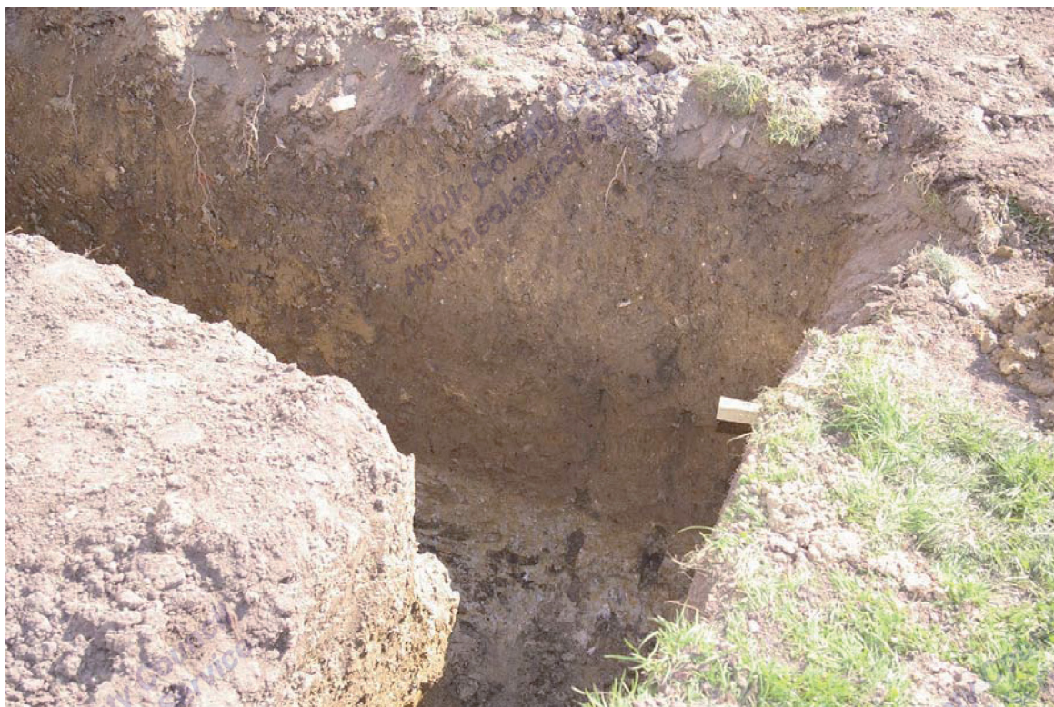
Figure 4. A view of part of the foundation trench for the proposed extension, showing the vertical section recorded in Figure 3 (looking south)
