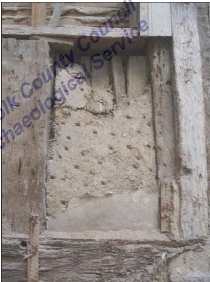
Figure 7. Wattle and daub panel revealed during renovation work.
