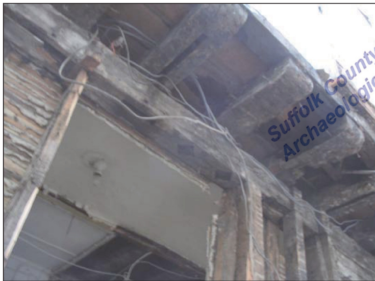
Figure 8. Sockets for former diamond window mullions and a mortice in the jetty plate for a former upright (window 1 on Fig. 6).
