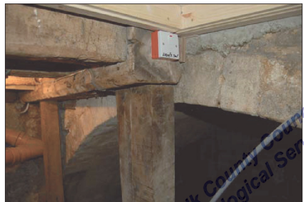
Figure 14. The timbers of the floor of the jettied building abut the vault.
