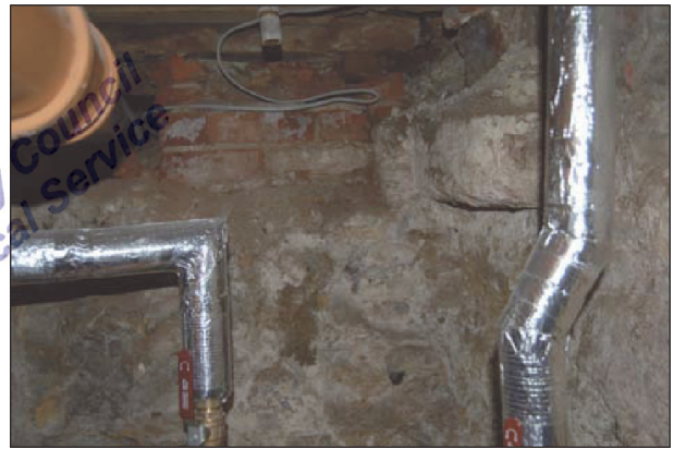
Figure 13. Step and rubble in the northeast corner.
