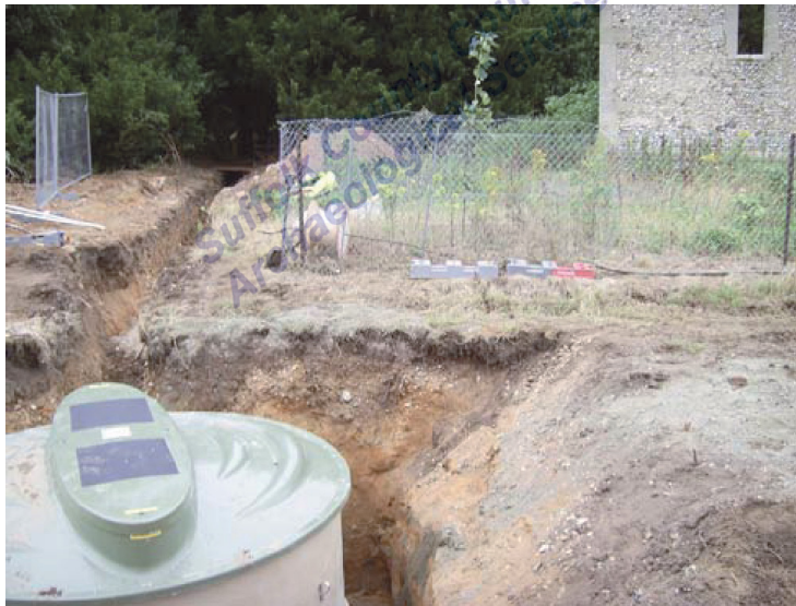
Figure 4. Sewage treatment unit with Fornham Church in the background.
