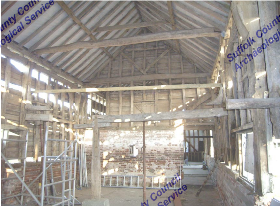
A2.7 General view of stable interior from west showing remains of removed ceiling with partition to barn in rear
