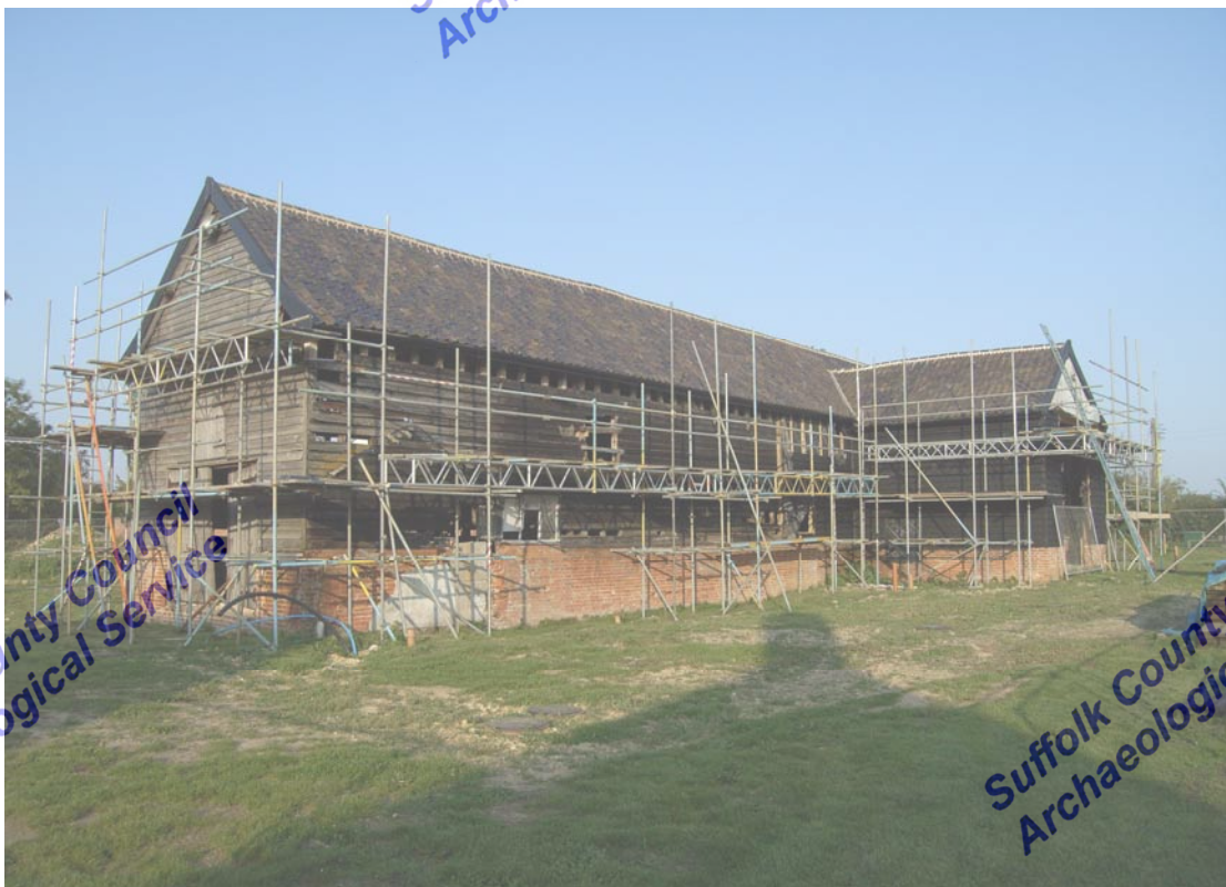
A2.2 Exterior from south-west showing roof scar of demolished southern shed to left
