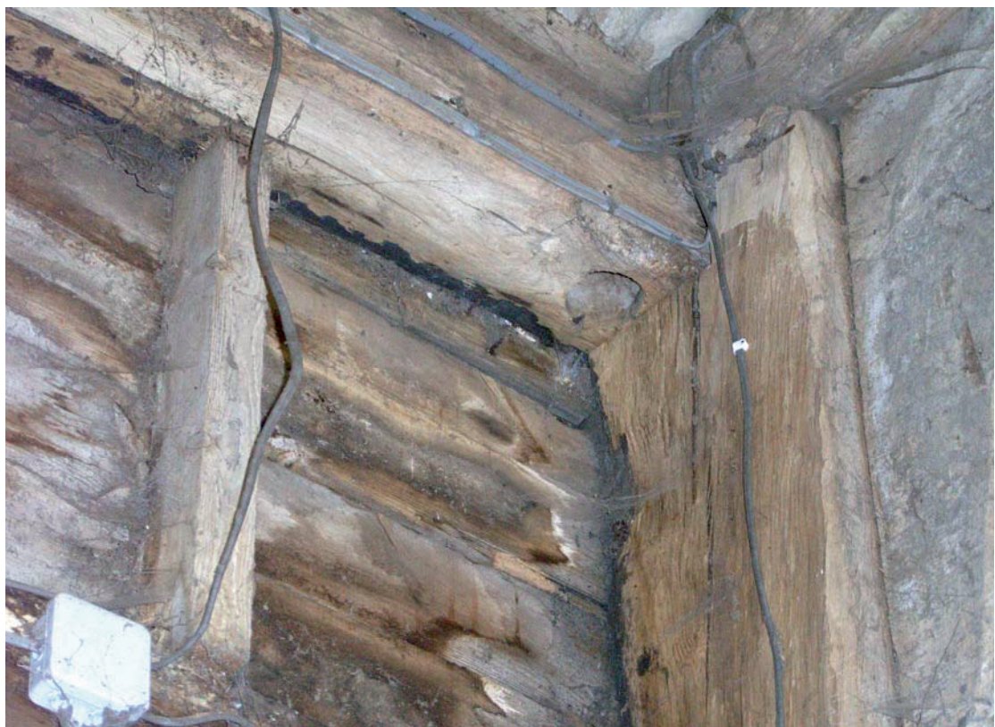
A2.6 Detail of roof-plate at southern end of central eastern bay showing circular housing for pin hinge of original door
