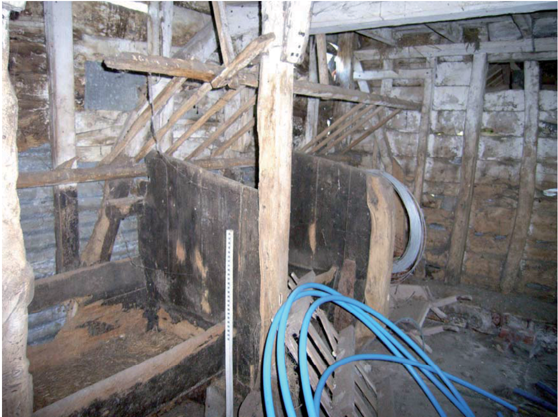
A2.3 Interior of timber-framed stable (3) showing low hay rack and manger with western gable to right
