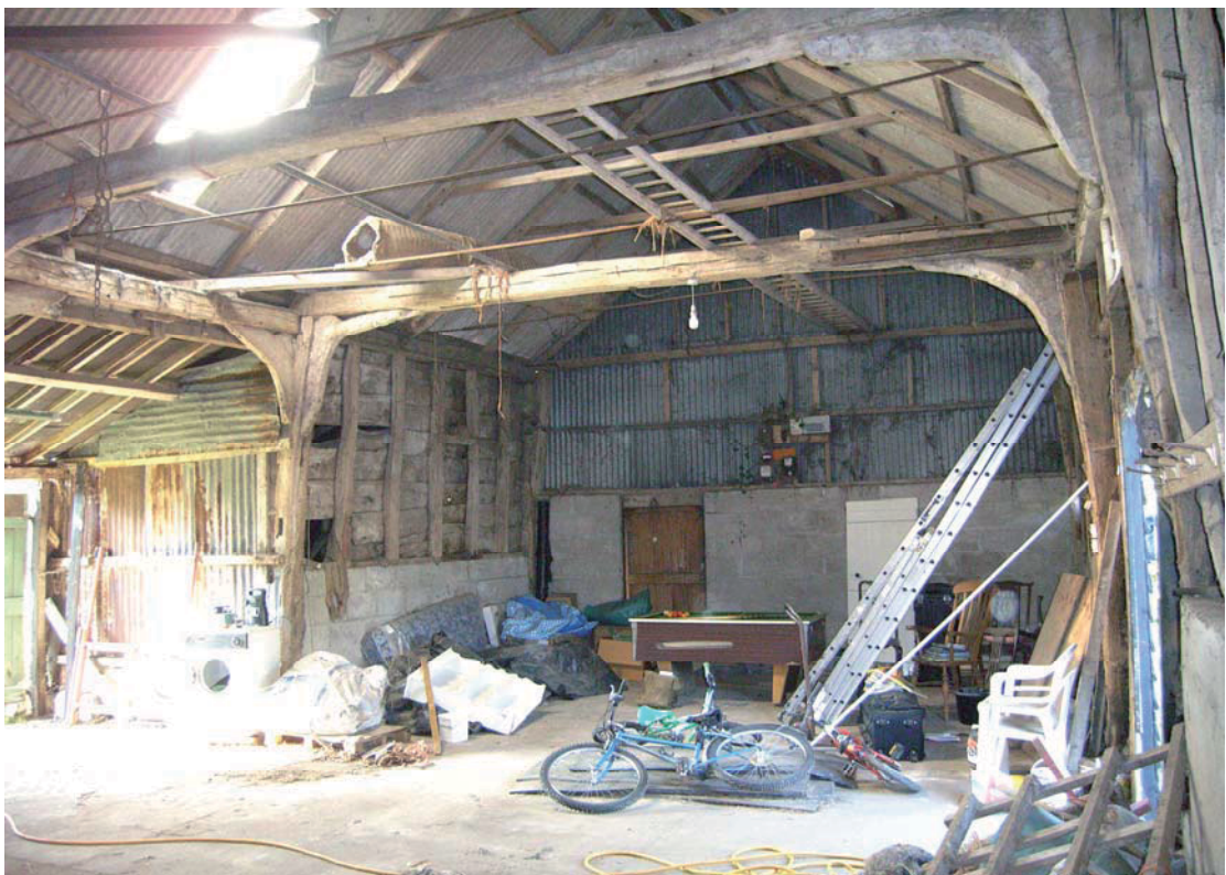
A2.4 Interior of Barn. General view from south showing rebuilt northern gable with western lean-to shed to left
