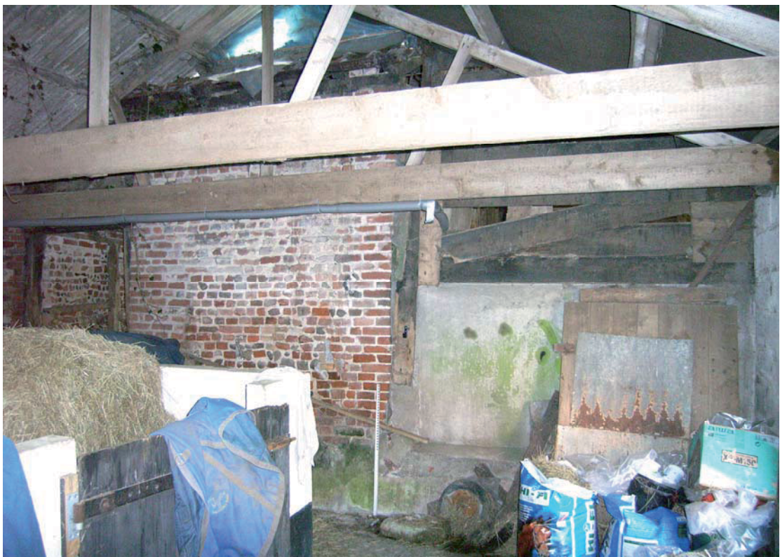
A2.8 Eastern external elevation of brick stable (2) from block-work stable showing original entrance door to left & southern bay of barn to right
