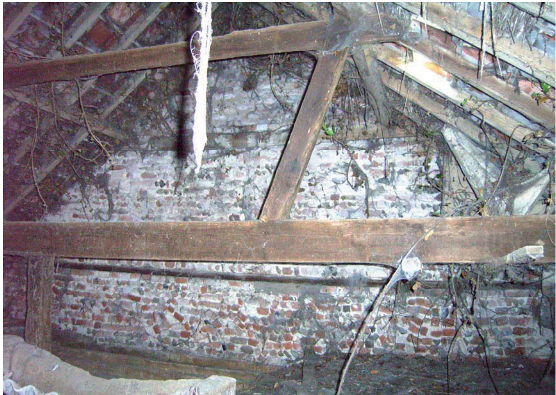
A2.8 Internal southern gable of brick stable (2) from hay loft showing softwood roof-structure
