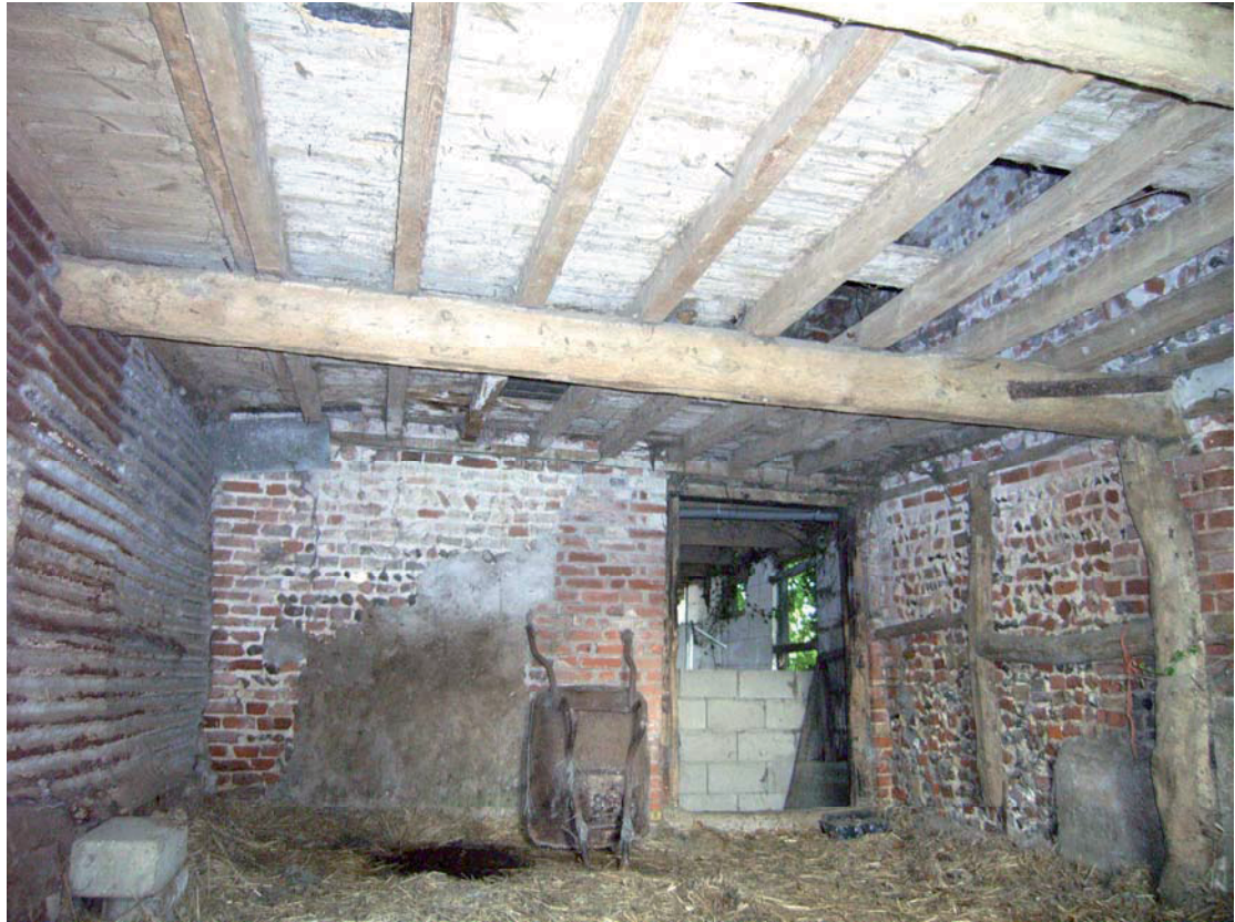
A2.9 Interior of brick stable from west showing hay loft ceiling and eastern entrance to right. The southern gable of the barn is shown to the left
