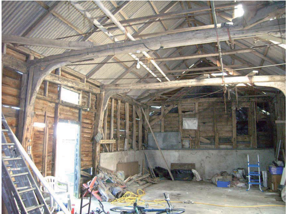
A2.5 Internal eastern elevation of barn from north showing original entrance in central bay to left and southern gable to right. The knee-braces replace original arch-braces
