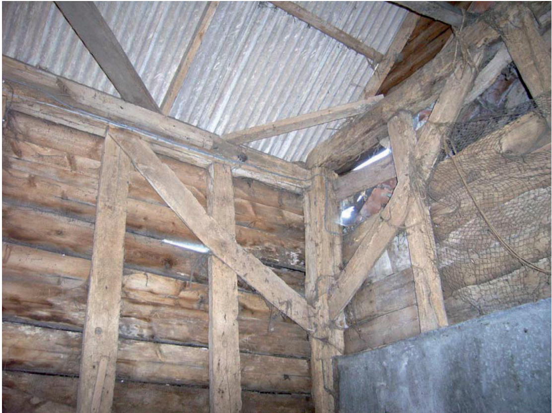
A2.7 Detail of original internally trenched wall braces in south-eastern corner of barn, showing southern gable to right
