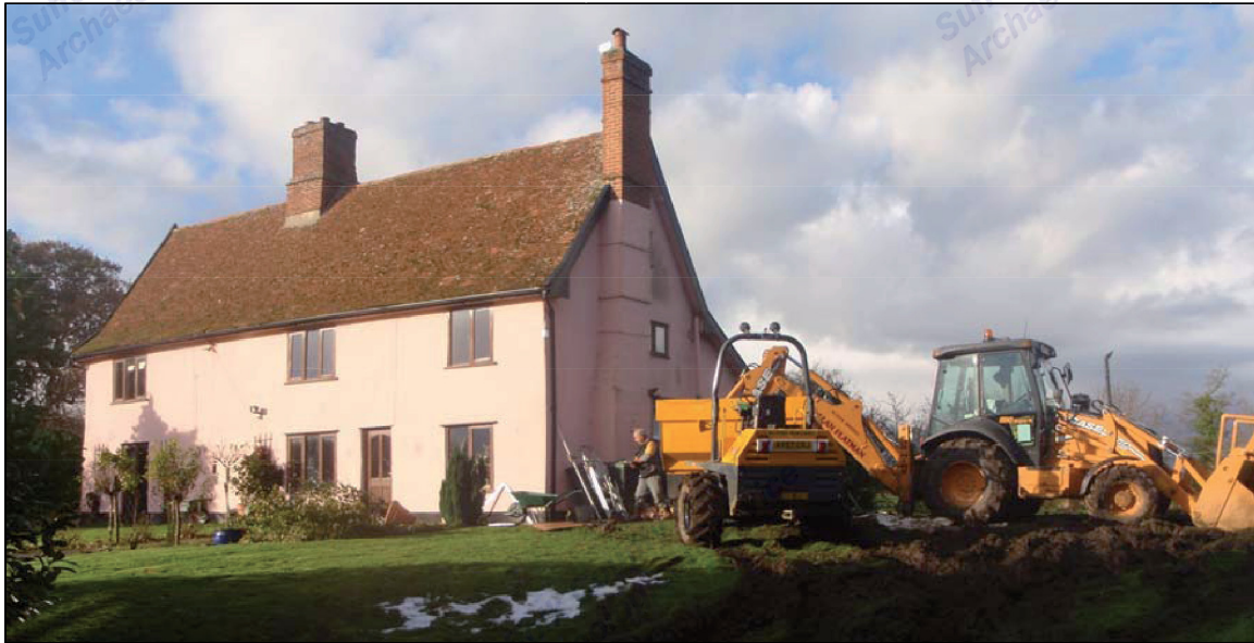
Plate I: general view of the excavation of the breakfast room footings, view looking north
