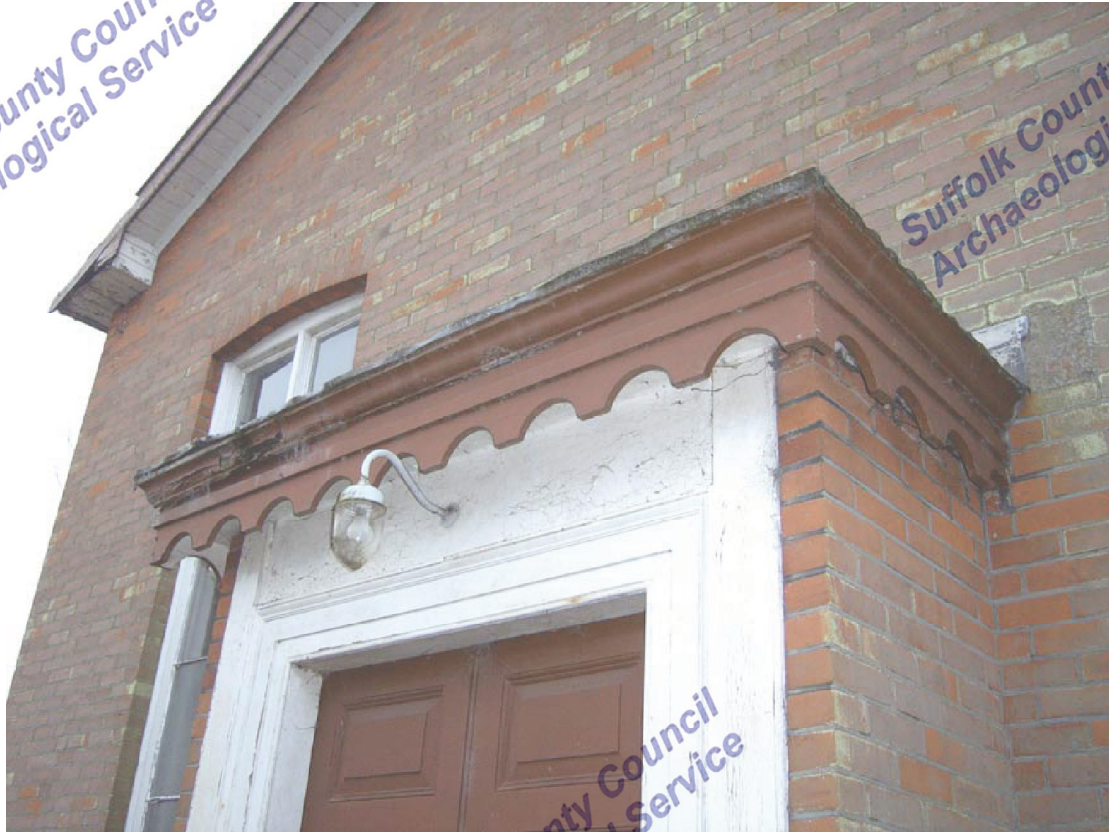
A2.3 Detail of original northern door and porch of 1843 showing decorated eaves board with early-20 th century brick cladding
